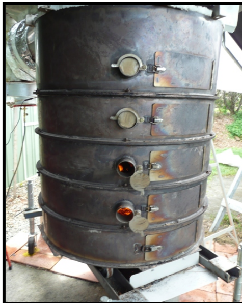
Photograph 37 - BiG gasification pilot plant
