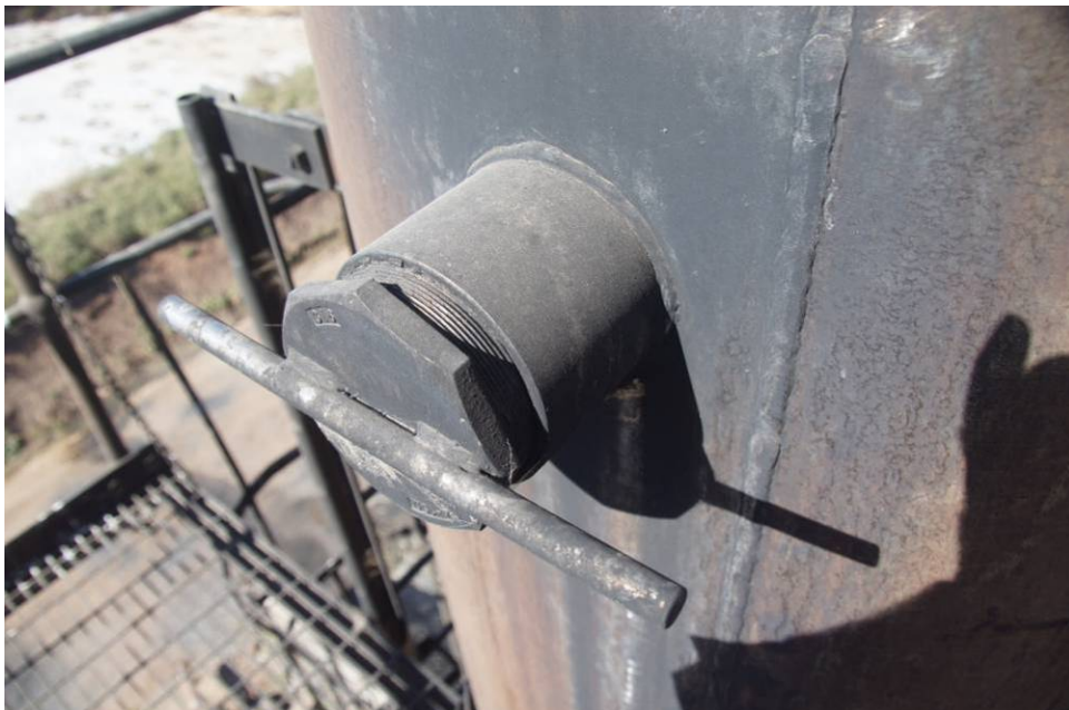
Photograph 29 – Sampling port on flue
