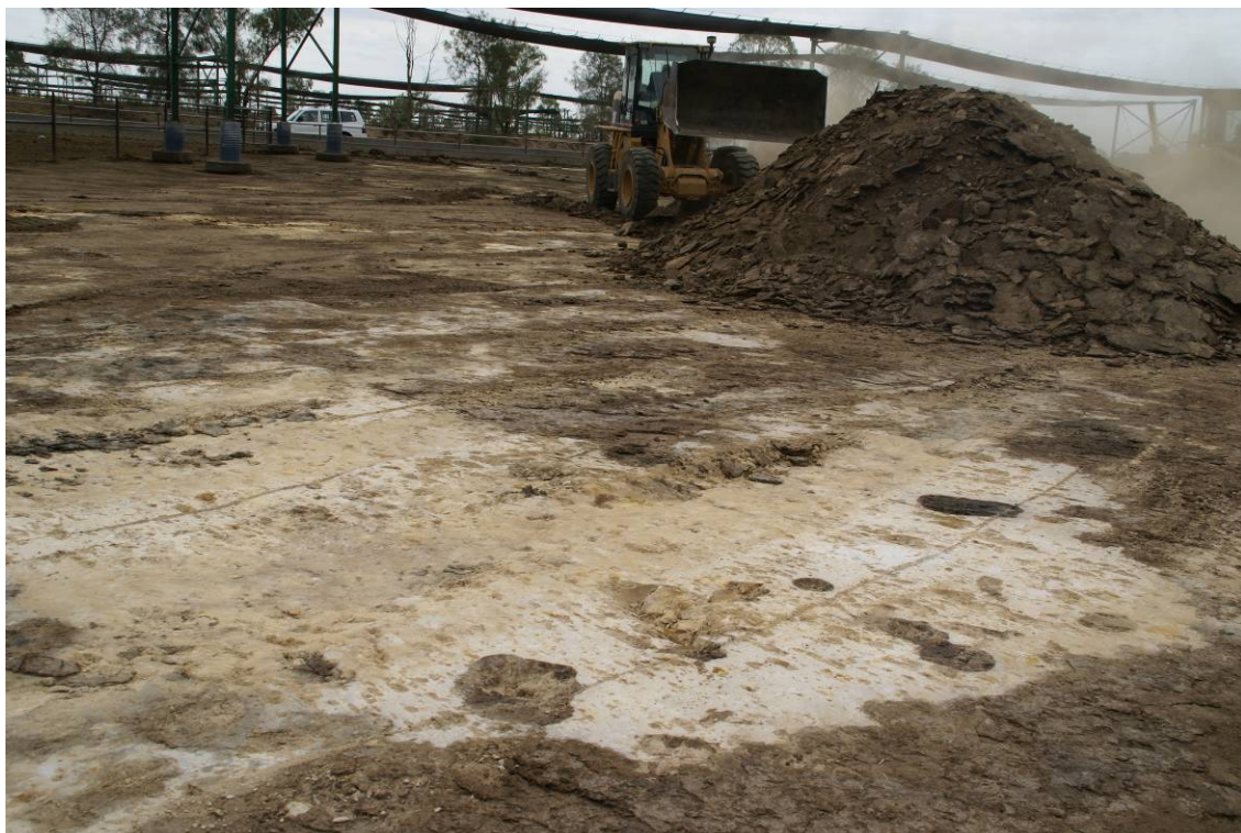
Photograph 6 – Pen cleaning with a front-end loader where the interface is removed exposing the clay base
