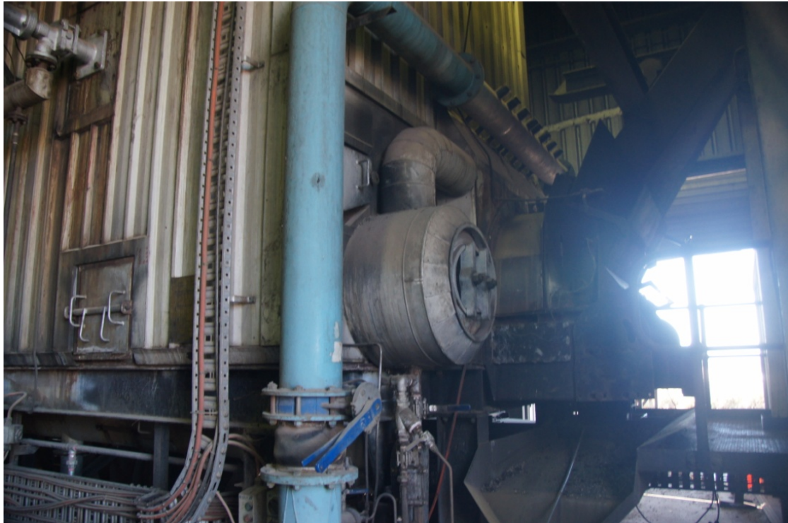
Photograph 26 – Coal feed into boiler
