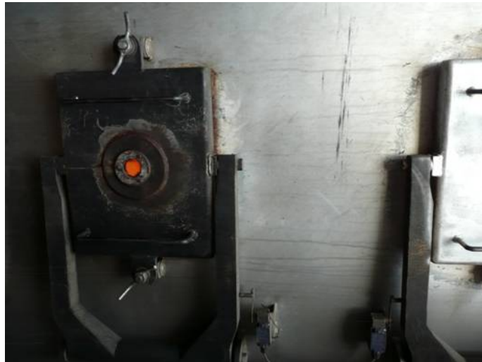
Photograph 15 – Boiler showing viewer port
