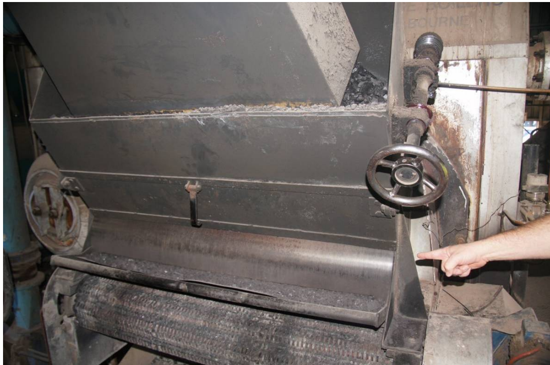
Photograph 27 – Chain bed and control gate on coal feed
