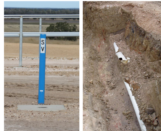
Marking and recording the location and depth of underground mainlines will prevent unnecessary and costly damage.
