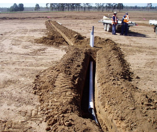
The PVC sleeve fitted over polyethylene pipe underneath the proposed concrete apron will make any replacement of the polyethylene pipe easier.
