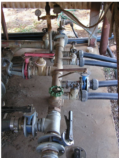
A pumped reticulation system manifold with various take-offs and shut-off valves for flow control
