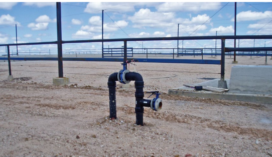
Shut-off valves allow individual troughs or rows of pens to be isolated without disrupting the water supply to other pens, or for purging pipes.
