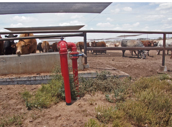
Isolation valves allow water supply to be cut off for repairs.
