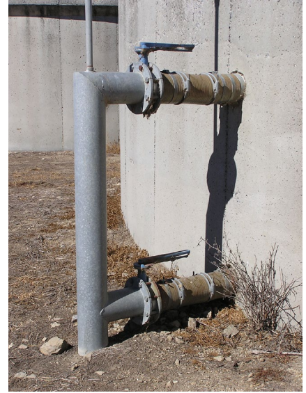
Galvanised steel mainlines have been largely replaced by PVC and polyethylene because of its workability, ease of repair and cost.
