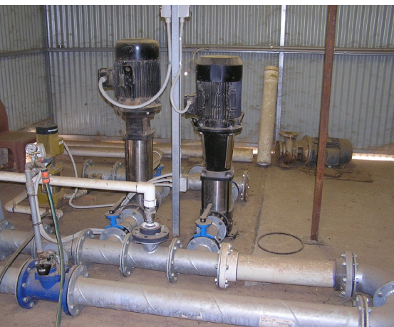
Pumped reticulation system with a standby pump and associated controllers and valving
