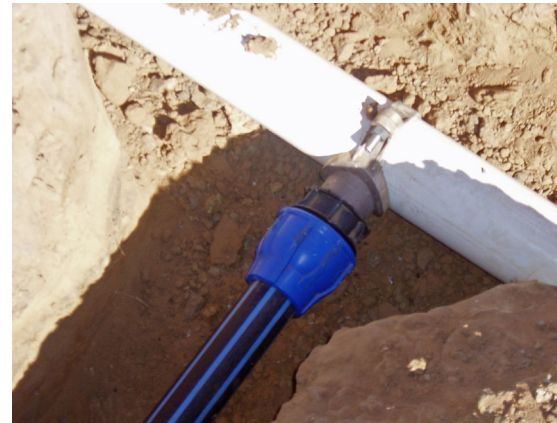
PVC piping is a common mainline material, easy to install and repair. This installation incorporates a polyethylene pipeline take-off to the trough. Polyethylene pipe is now available in larger diameters (100 mm plus).
