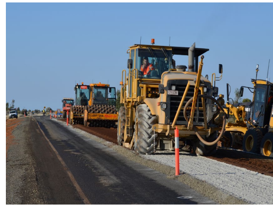
Stabiliser machine mixing binder agent into road base material. The mixed material is being compacted immediately by the sheepsfoot compacters.
