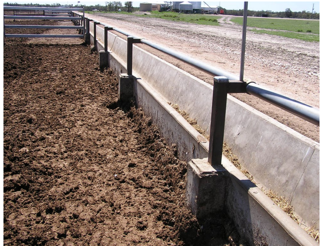
Intruding posts will make apron cleaning difficult.
