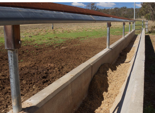
Posts cast into the concrete wall need to be treated with epoxy to prevent corrosion at the concrete joint.
