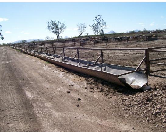
Bunk of corrugated steel half-pipe inside which rubber belting has been subsequently laid. Same issues as above.
