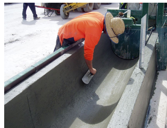
Feed Bunk G. The slip-form machine runs on prefixed rails, then the surface is steel trowelled.
