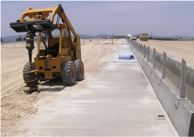
Concrete apron on the pen side of the bunk provides a stable base against mud holes, and allows easy cleaning.
