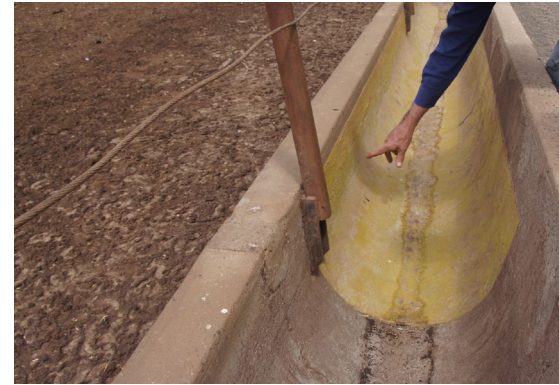
Sealing the inside of the feed bunk with epoxy resin will protect the surface from chemical attack and abrasion.
