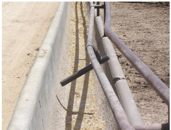
Posts cast into the back wall can corrode and be damaged.
