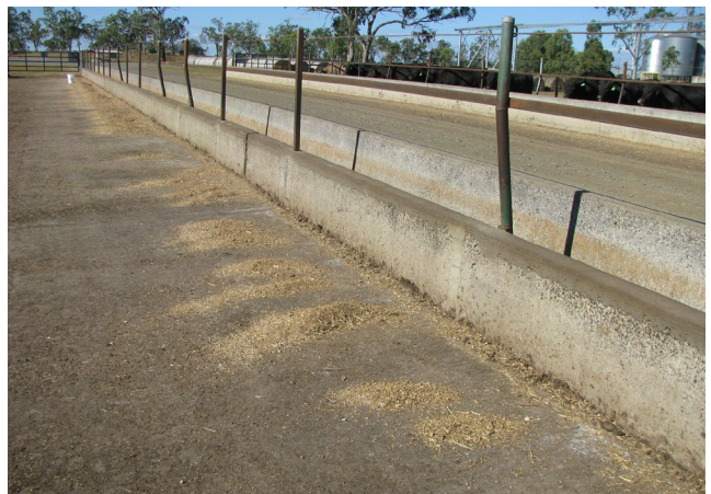
Posts cast into the bunk back wall of the feed bunk can rust at the joint between the post and the back wall. Replacement posts bolted inside of the bunk could inhibit bunk cleaning.
