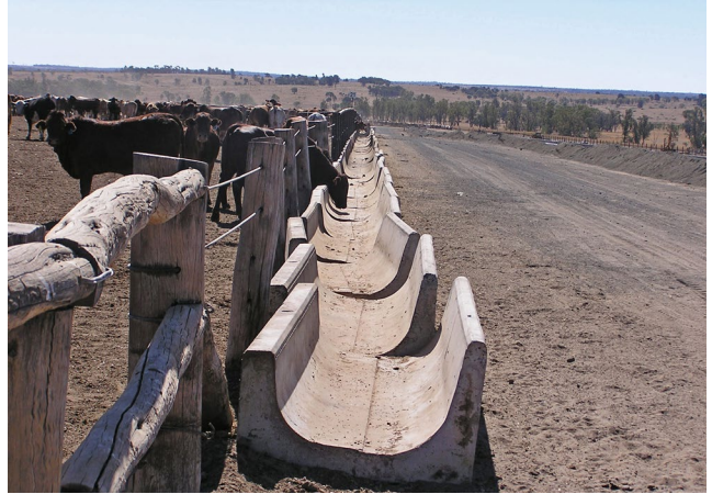
Without suitable anchoring, pre-cast bunk sections can be moved out of alignment.
