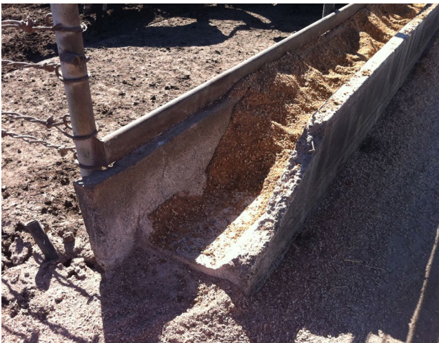
Damage to the ends of feed bunks by feed trucks will be minimised with a straight feed road and placing a steel bollard.
