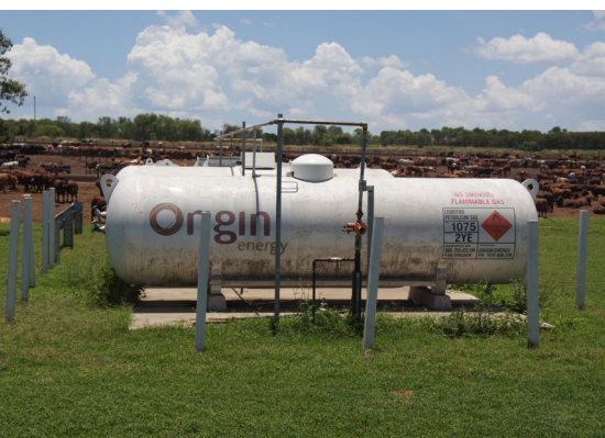
LPG tanks with bollard protection from potential vehicle impacts.
