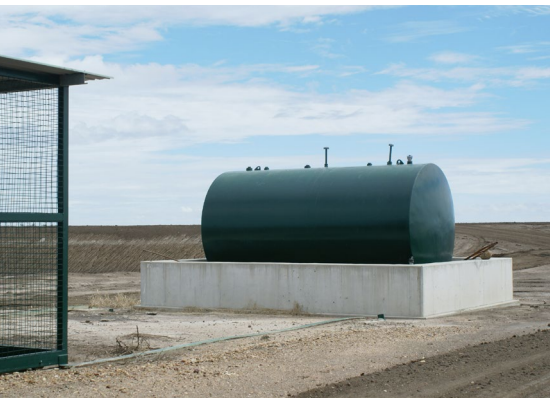
Diesel tank with a good paint coating, free from rust and damage. A more reflective colour (silver or white) would be preferable.
