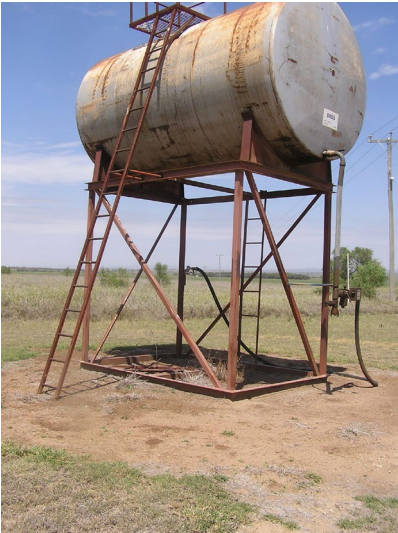
Rust – tanks should be protected against corrosion by a good paint coating.
