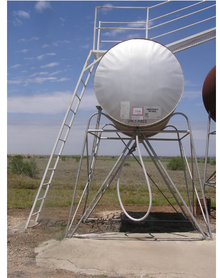
Four legs on support structure with braces close to their base, legs and bracing straight, in good condition and securely attached. Ladder sound and secure, all rungs present, suitable hand holds near ladder.
