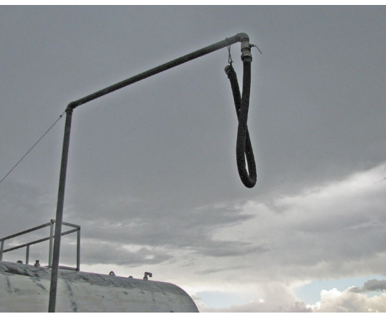
Fittings, pumps and hoses – fuel dispenser hoses must be of an approved type for the fuel, with an internal bonding wire for dissipating any static electricity charge generated during dispensing.
