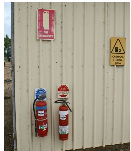
Clearly signed fire extinguishers on the outside of storage
