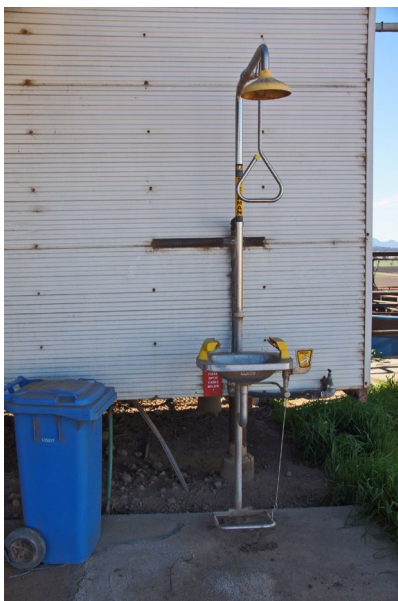
Emergency shower and hand basin located outside of chemical store.
