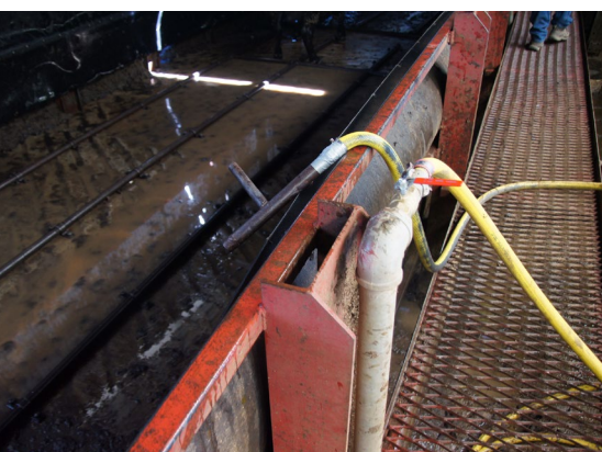
Adjacent catwalk with high pressure hose and nozzle
