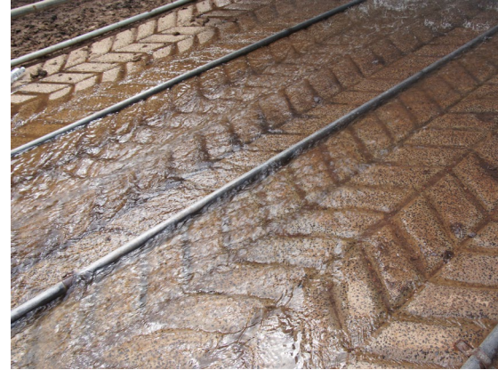
Concrete floor with herringbone pattern and above floor water pipework. Drainage flow is parallel with pipework.
