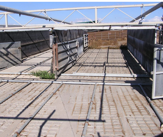
Side by side soaking pens with above-floor pipework and an overhead spray system
