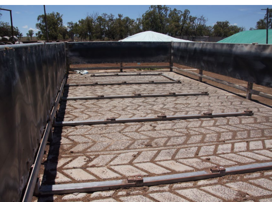
Concrete floor draining from right to left with herringbone pattern across the yard. This yard has rubber sheeting on fences and uses RHS steel for water delivery, with nozzles protected by welded covers.
