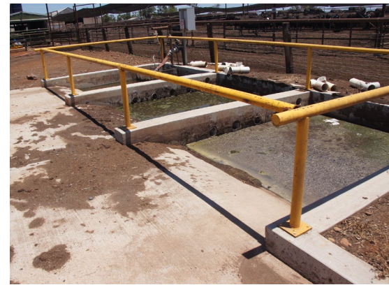
Triple-bay trafficable sediment trap. Drainage water can be directed to other basins to allow sediment to dry out.
