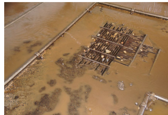
Above ground pipes may restrict the flow of water to the drainage pit.
