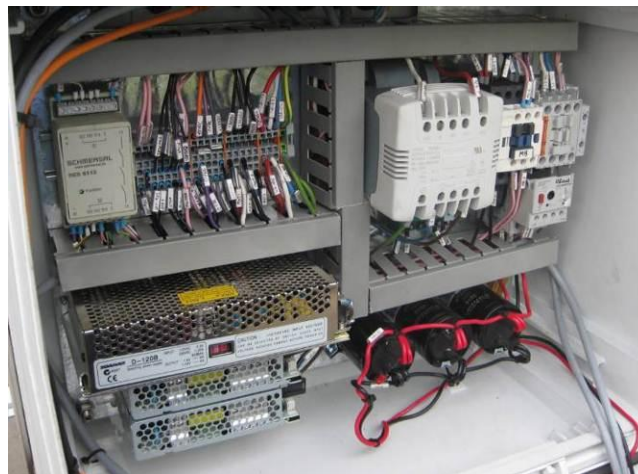
Fig.9 View of the electrical panel on the ACC saw.
