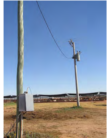
Overhead electricity – supply with aerial transformer and sub-board
