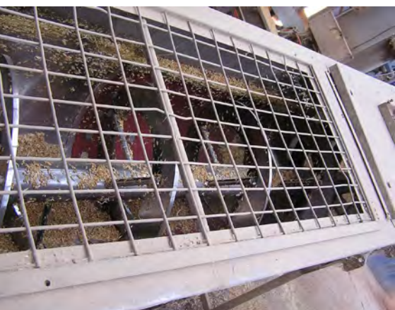
An open spiral mixing auger to convey and mix the grain from the storage silo past the grain-wetting station to the tempering silos.
