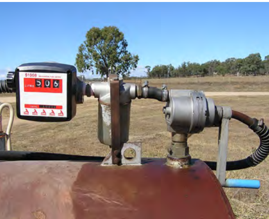
Fuel hose in good condition, with fuel filter and meter to record fuel usage.
