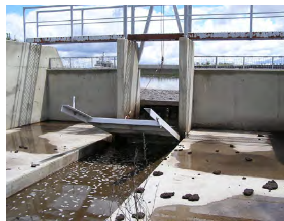
A drop weir structure on a sedimentation basin relies on human intervention for use. Thus the operation of the system can be stalled if workers cannot reach the sedimentation system as during flooding.
