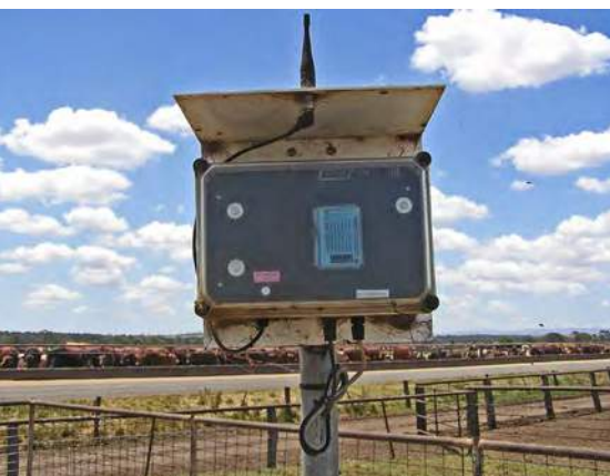
AWS with radio link to office.
