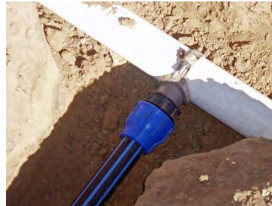
PVC piping is a common mainline material, easy to install and repair. This installation incorporates a polyethylene pipeline take-off to the trough. Polyethylene pipe is now available in larger diameters (100 mm plus).
