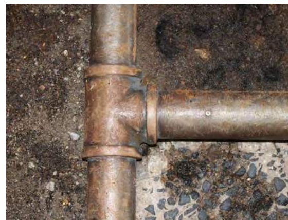
Holes drilled in pipes create a quick and cost effective spray system.
