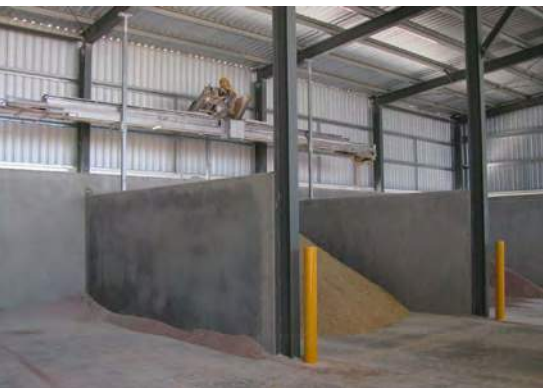
A cross conveyor can transfer grain into one or more bays. Highly visible bollards protect structural members and walls from damage by machinery.
