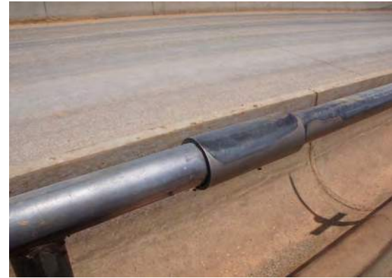
Expansion joints prevent buckling of steel cattle restraint in hot weather.
