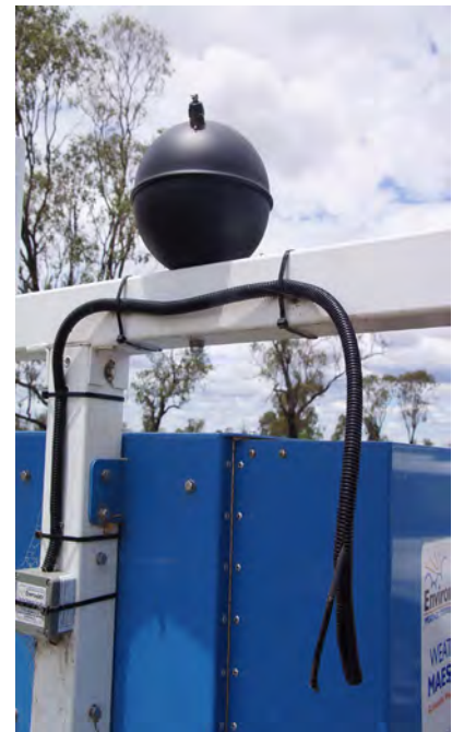
Well protected cabling on an AWS.
