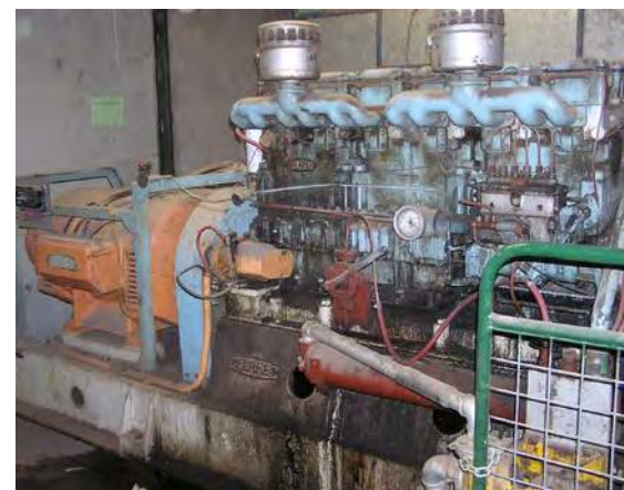
Diesel engine-powered backup generator housed inside shed
