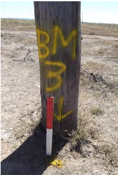
A poorly located Temporary Bench Mark (TBM) sited near to infrastructure not affected by earthworks.
