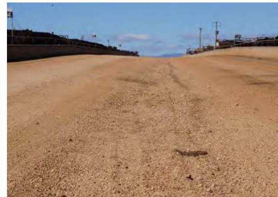
Road cross section – back to back layout with cross-fall to centre of the feed lane and longitudinal fall along the road
