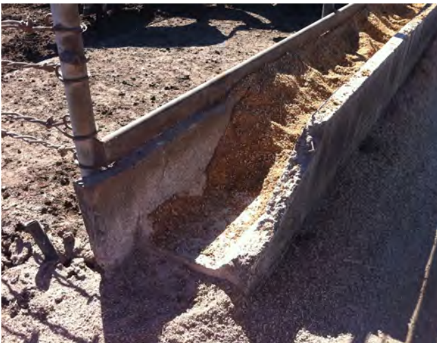
Damage to the ends of feed bunks by feed trucks will be minimised with a straight feed road and placing a steel bollard.
