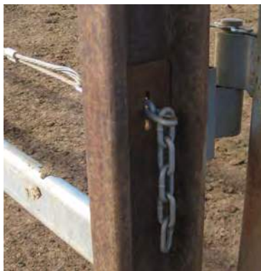
Cable tension is achieved and maintained by locking the cable in the railway line using chain links.
