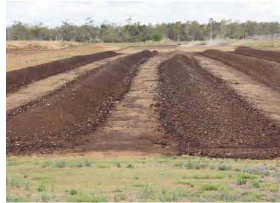
Composting areas also need an impervious base and an even slope of 1–3%.
