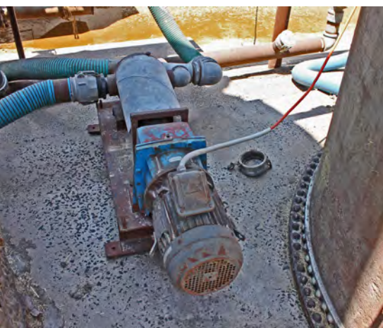
Handling equipment should be of adequate size to deliver the liquid to the delivery point. Larger diameter pipes are required for viscous feedstuffs, such as molasses.
