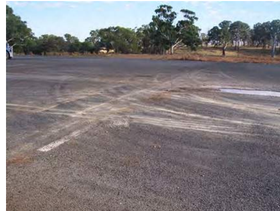
Markers embedded into paving as a guide for reversing vehicles
