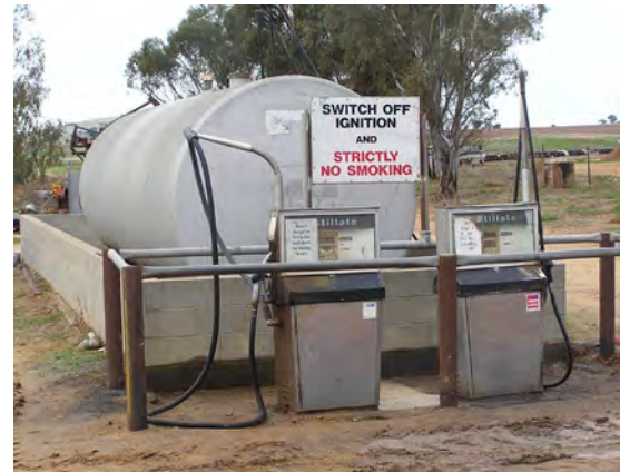
Diesel and petrol fuel storage with bowlers. Bunding behind and to each side of the facility is effective against spills; however it could fill with water after rain and has to be drained.
