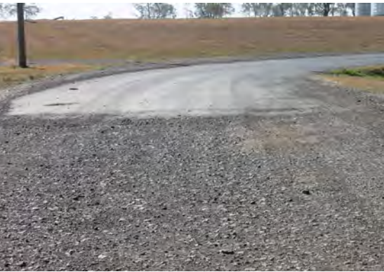
Gravel loss and structural issues are most common on road curves where shear stresses from vehicle loadings are the highest. Bitumen seal on road curves reduces road maintenance but potholes can form easily at the transition with the unsealed section.
