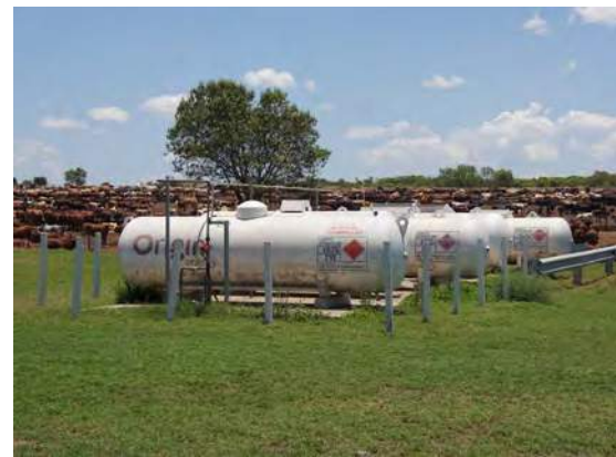
Banked LPG storage tanks – with bollard protection
