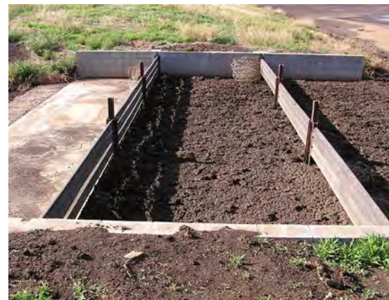
Horizontal timber slat control weir showing deposited sediment on the upstream side with little manure on the downstream side. The basin has drained completely and is drying out so that the solids can be removed.
