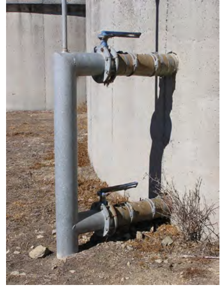
Galvanised steel mainlines have been largely replaced by PVC and polyethylene because of its workability, ease of repair and cost.
