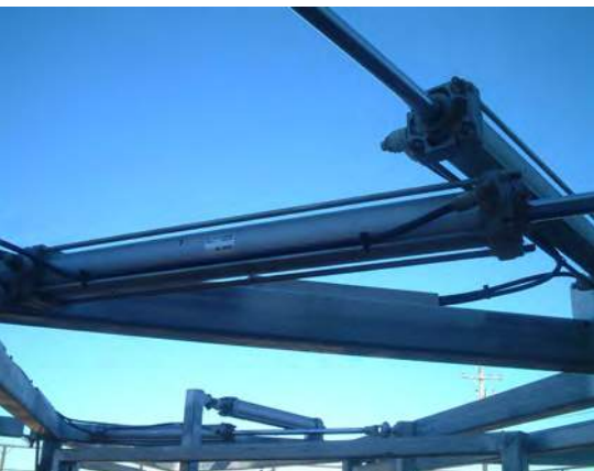
Power-assisted pneumatic gate
