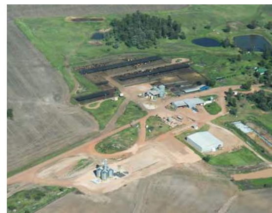
Feedlot undergoing expansion. The old feed preparation and storage area is next to existing pens and a new feed mill is being constructed central to both new and old pens.
