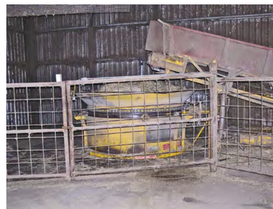
A permanently positioned electric powered tub grinder with the discharge conveyor set below ground level. This arrangement inside the commodity shed presents a greater fire hazard than a portable self contained unit that is easy to access and clean down.
