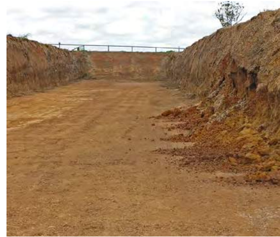
Hillside pit with near vertical walls. Side walls that are too steep may collapse on impact of machinery, or from erosion when empty.
