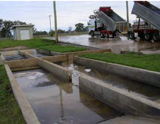
Quadruple trafficable sedimentation basin side by side arrangement. Wastewater is diverted into one or more bays.
