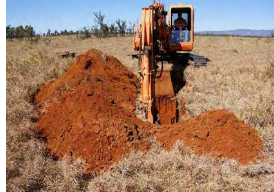
Test pit excavation. Separate the soil horizons or changes in soil texture during excavation to allow soil samples to be collected from each type of material encountered.
