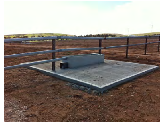
Aprons allow cattle to access to the trough under all weather conditions and allow access for cleaning (Position A).
