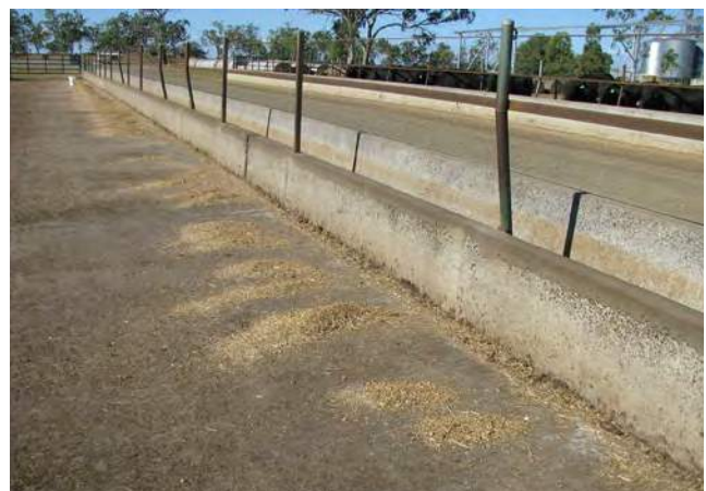
Posts cast into the bunk back wall of the feed bunk can rust at the joint between the post and the back wall. Replacement posts bolted inside of the bunk could inhibit bunk cleaning.
