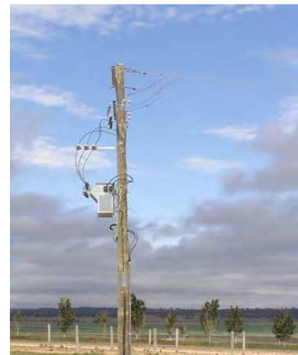
Overhead electricity – supply pole and transformer
