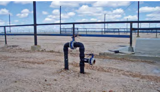
Shut-off valves allow individual troughs or rows of pens to be isolated without disrupting the water supply to other pens, or for purging pipes.
