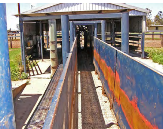
Steel frame structure over crush with half-sheeted walls. Sharp contrast between dark shadows and bright sunlit areas could make cattle baulk.
