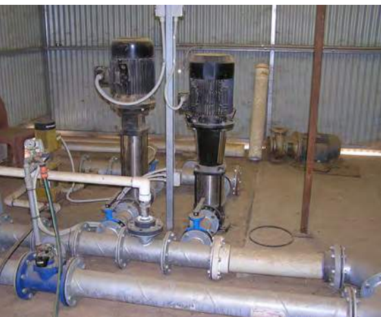
Pumped reticulation system with a standby pump and associated controllers and valving
