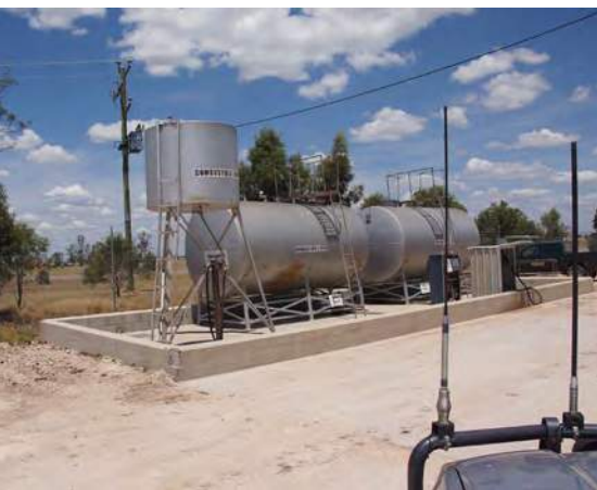
Impervious bunding around fuel storage tanks must be large enough to contain the combined capacity of the tanks plus 20 minutes of fire-control water.
