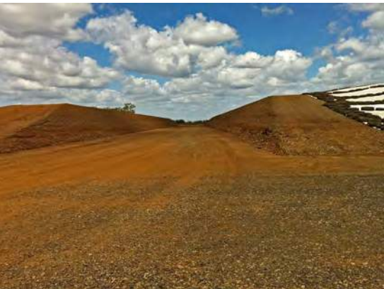
Open-ended, above ground bunker with compacted gravel base and clay walls. The walls are trimmed to the design batter and base to the design grade. A flat sloping end face allows water to drain from top of wall to ground level without eroding the face.
