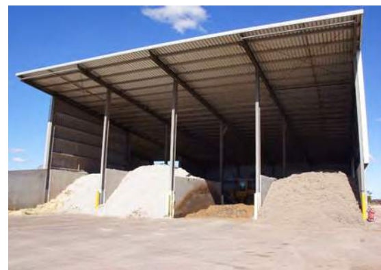
A purpose-built, stand-alone commodity storage shed. The high roof allows direct loading of storage bays from a tipping-trailer truck. A large concrete apron in the front of the bays allows easy vehicle manoeuvring.
