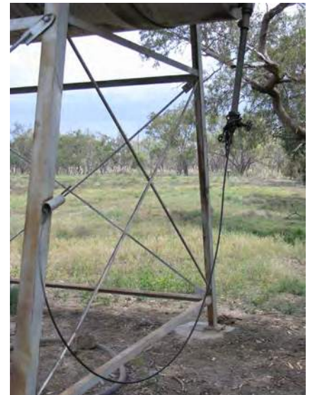
Feet pads above ground and secured to concrete pad with well-braced legs.
