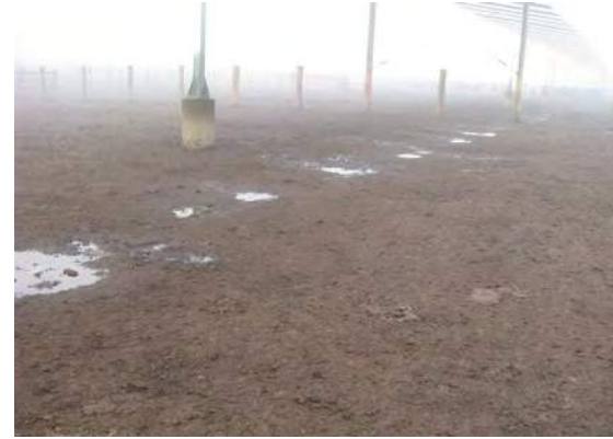
Corrugated iron sheets can concentrate rainfall runoff to localised areas; ponding will damage the pen surface.
