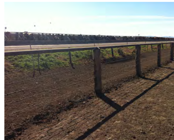
Good quality timber is becoming difficult to source. A steel capping rail will prevent posts without concrete footings from leaning under pressure from cattle.
