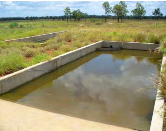
Dual trafficable sedimentation basins allow one to be taken offline to enable sediment to dry. Separate basins cost more than a side by side arrangement. These basins are adequately sized for cleaning machinery but do drain to bed level.
