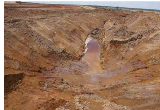
Problems may arise during construction earthworks. Groundwater encountered will need appropriate drainage.
