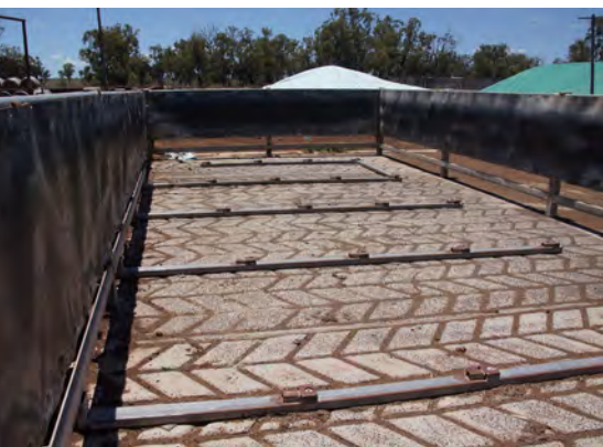
Concrete floor draining from right to left with herringbone pattern across the yard. This yard has rubber sheeting on fences and uses RHS steel for water delivery, with nozzles protected by welded covers.
