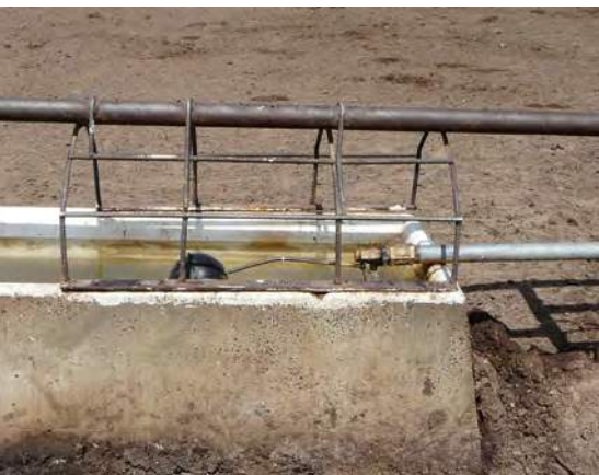
Steel cage to protect float
