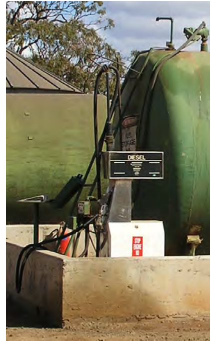
Fuel type identification and easily accessible fill point
