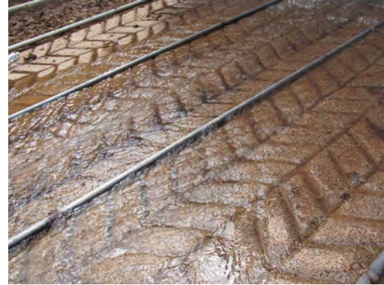
Concrete floor with herringbone pattern and above floor water pipework. Drainage flow is parallel with pipework.
