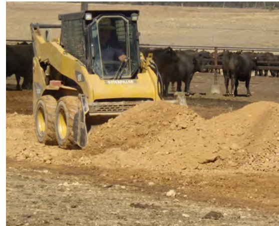
Poorly graded material being used in pen repairs – note the large percentage of fines.
