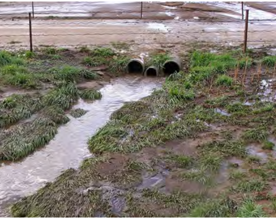
Use the ratio of rainfall to surface runoff (runoff coefficient) to calculate for adequate drainage.
