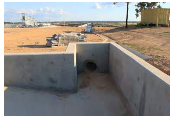
Trafficable sedimentation basin with offset weeping wall/bar screen segment. Wastewater drains to bed level.
