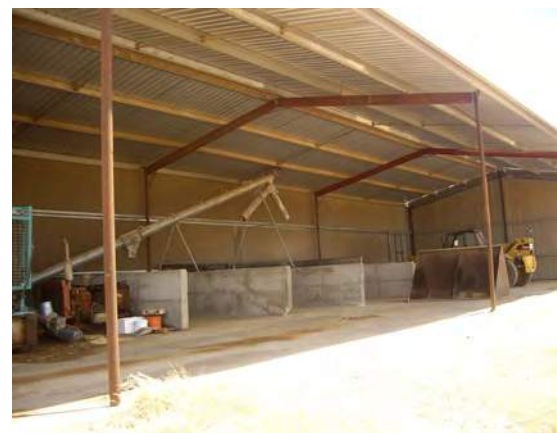
Any storage facility may be adapted to store feed commodities. The side wall from this machinery shed has been removed and storage bays constructed.
