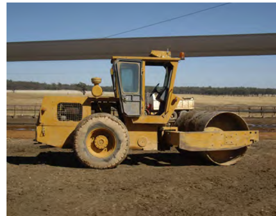
Smooth-drum rollers are used to compact the high spots until the surface is smooth—usually after a grader has levelled the surface.
