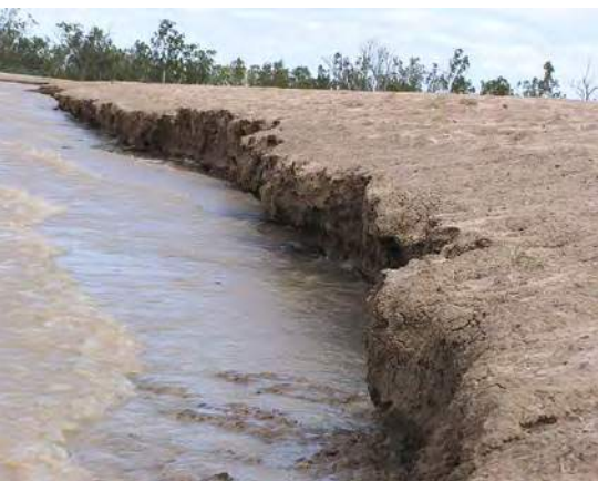
Lack of vegetative cover and a highly dispersive soil allow wave action to erode this internal batter.
