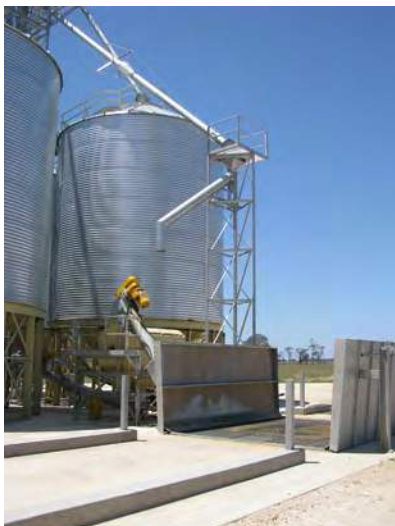
A drive-over receival grid with raised covering doors. A screw conveyor transfers grain from the hopper to a grain conditioner or scalper.
