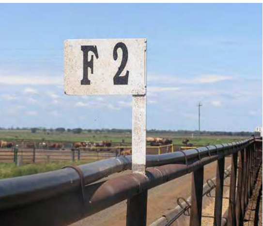
Drinking water can become extremely hot if steel or plastic water pipes are exposed to solar radiation.
