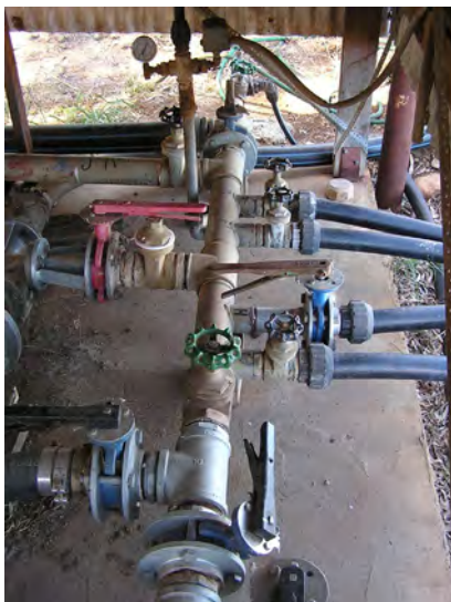
A pumped reticulation system manifold with various take-offs and shut-off valves for flow control
