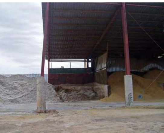
Concrete placed around structural members offers little protection, as the impact is transferred directly to the steel member.
