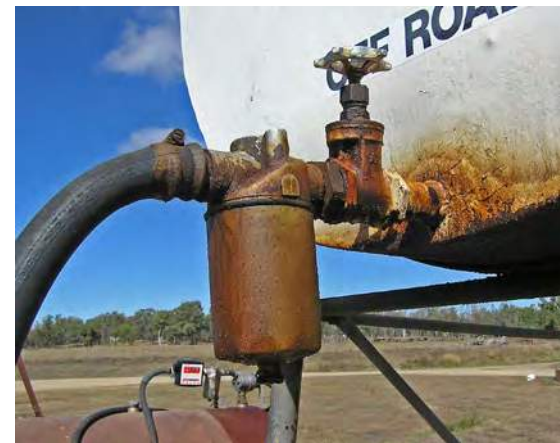
Isolation valve on dispenser is kept turned off except when dispensing fuel. Rust on the tank and outlet pipe needs to be treated.
