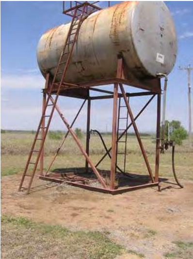
Rust – tanks should be protected against corrosion by a good paint coating.
