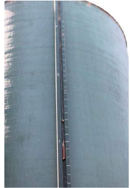
Level indicator fixed to the outside of a storage tank allows inventory levels to be easily checked and recorded.
