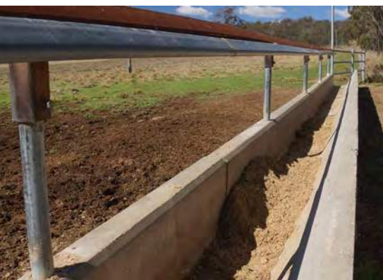
Posts cast into the concrete wall need to be treated with epoxy to prevent corrosion at the concrete joint.
