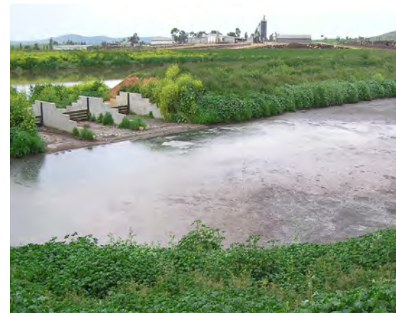
Upstream of the outlet control structure. Excessive removal of sediment has caused the floor of the basin to be lower than that of the control structure so the basin cannot fully drain. When removing sediment, do not alter the base of the sedimentation structure.
