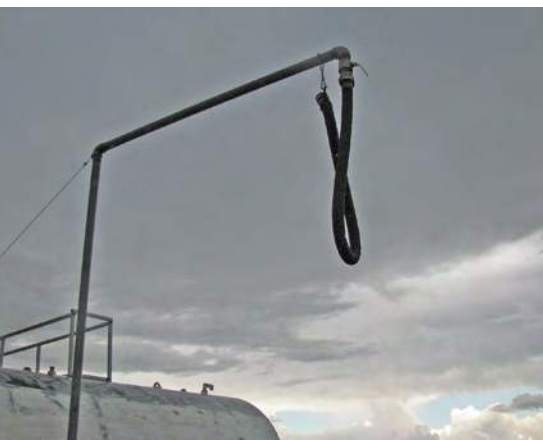
Fittings, pumps and hoses – fuel dispenser hoses must be of an approved type for the fuel, with an internal bonding wire for dissipating any static electricity charge generated during dispensing.
