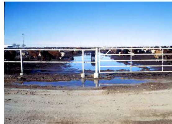
With very flat pens, pen to pen drainage may form in the middle of the pens.
