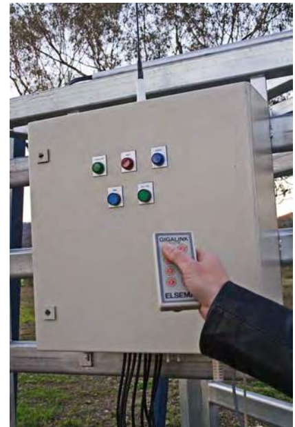
Controls for operation of gates from hand-held remote.
