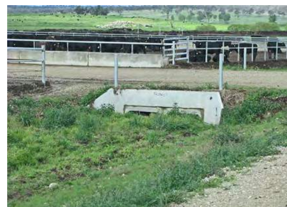
Sediment is deposited when vegetation reduces stormwater flow through culvert.
