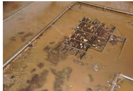
Above ground pipes may restrict the flow of water to the drainage pit.
