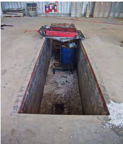
Inspection pit with stairs for access. Pit should have temporary fencing when not in use.
