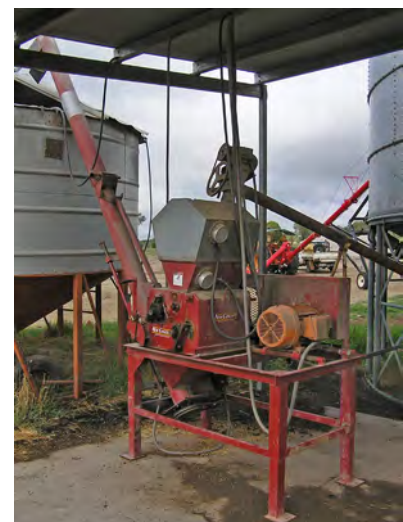
A single electric belt-drive roller mill. Grain is conveyed to the hopper above the rollers and then to a holding bin.
