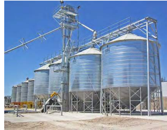
Receival grid, grain handling and cone-bottom silos. The grain is conveyed from the receival grid to a bucket elevator, with gravity fall to a horizontal conveyor for transport to the silo of choice. The height of the bucket elevator is reduced by using a horizontal silo loading conveyor.
