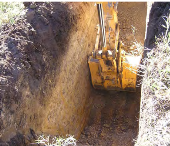
Geotechnical information of the site is gained by excavating test pits, sampling and analysing the engineering properties of the soil material.
