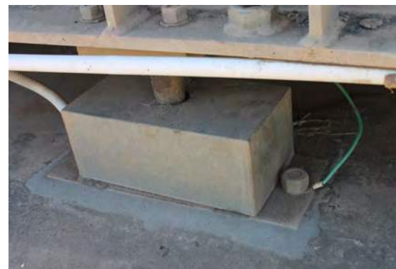
Load cell and weighbridge located above ground allows easy access for maintenance and re-calibration, and good drainage.
