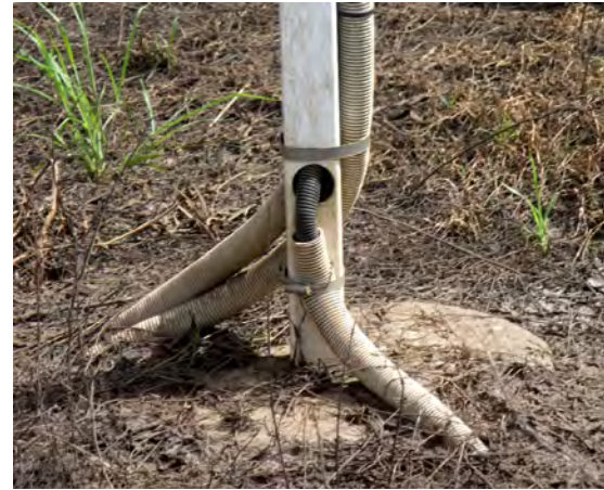
All cables to and from the AWS need to be protected from damage by machinery and animals. Cockatoos and rodents chewing on exposed cables lead to loss of data and expensive repairs.
