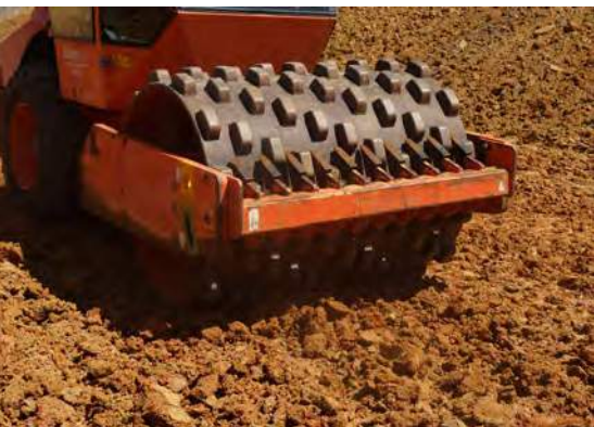
Clay liners should be compacted with at least eight passes of a sheepsfoot roller.
