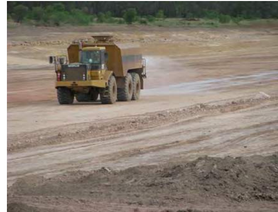
Dry surfaces may need spraying with water to allow the required degree of compaction.
