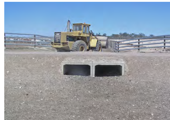
This concrete box culvert allows cleaning of settled manure in the drain on both sides of the culvert.
