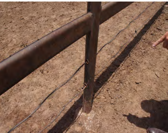
Cables passing through steel fence posts need a steel sleeve to reduce fraying. Sleeves prevent water entering the hollow post but can accumulate moisture which accelerates corrosion of the cable. This is an expensive fabrication technique.
