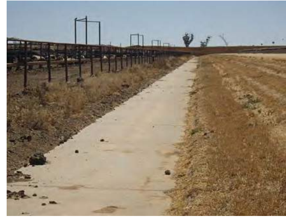
A well-maintained concrete drain within a feedlot. The dimensions of this drain allow access for cleaning equipment.
