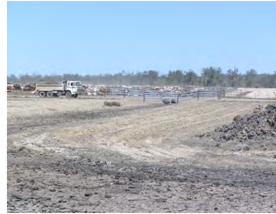
A view upstream of the sedimentation system showing the drainage line from the pens to the sedimentation system. The drains run under an on-site roadway, through a concrete culvert that permits the uninterrupted flow of effluent to the sedimentation system.
