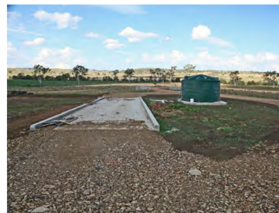
This concrete pad is of suitable length, but too narrow. Water is supplied, but the pad is flat and there is no controlled wastewater drainage system.
