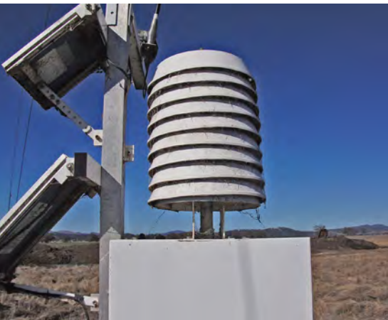
Spider webs and dust may affect the ventilation of humidity and temperature sensors within the screen.
