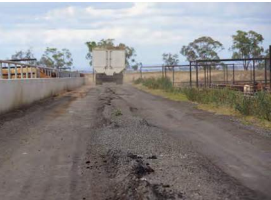
Rutting on a sealed road with poorly prepared subgrade.
