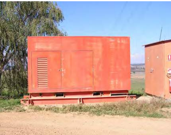
Self-contained backup generator on skid-mount
