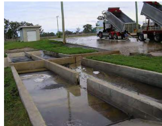
A double-sided trafficable solids basin at a truck wash facility
