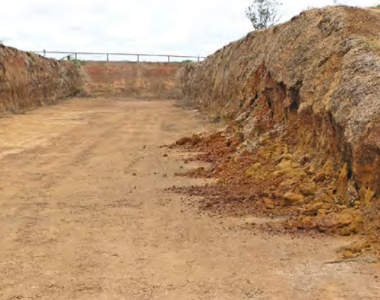
Batters that are too steep for the soil type and strength will collapse.
