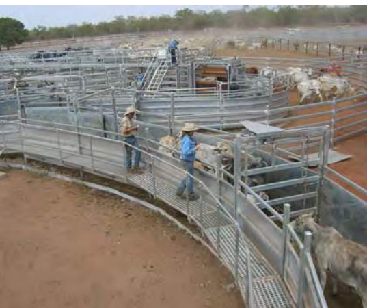
Curved races encourage steady movement of cattle. Operator safety is promoted by external walkways that separate cattle and handlers.
