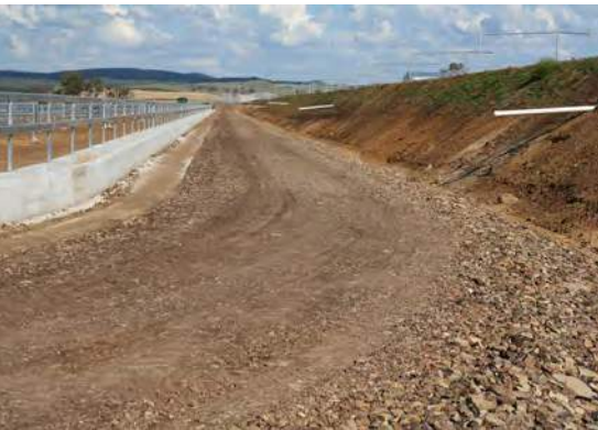
Coarse-graded material used in road construction— larger stones have been graded to the shoulder.
