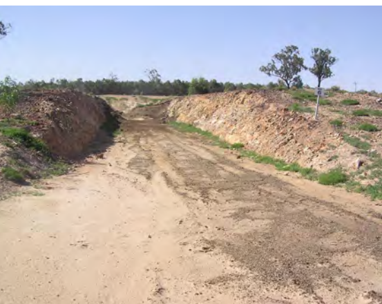
A pit excavated into gently sloping site. Cut soil material has been used to raise height of the embankment, but contains rocks.
