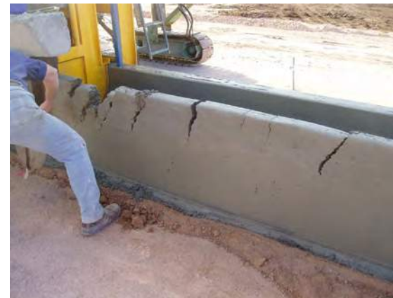
Good concrete mix with consistent moisture content is essential throughout the whole slip-form process—or problems will occur.
