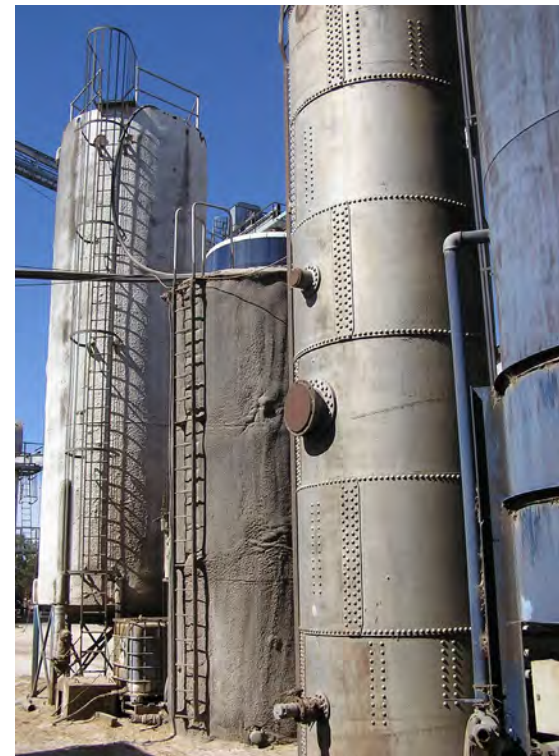
A bank of conical and flat-bottom steel tanks. Filling point is easily accessible at ground level, or at the base of conical tanks. Note there is insulation on some tanks to keep liquid warm and reduce viscosity.
