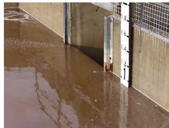
Marker indicating sediment buildup. The level of buildup can be seen when water is released through the drop weir.
