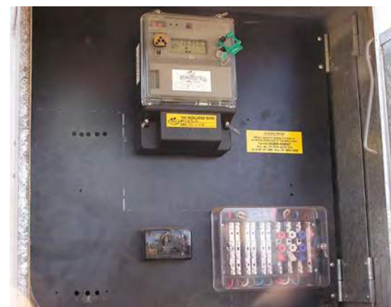
Power Authority meter – solid state with LCD display
