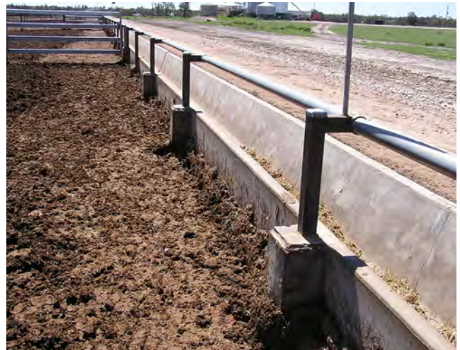
Intruding posts will make apron cleaning difficult.
