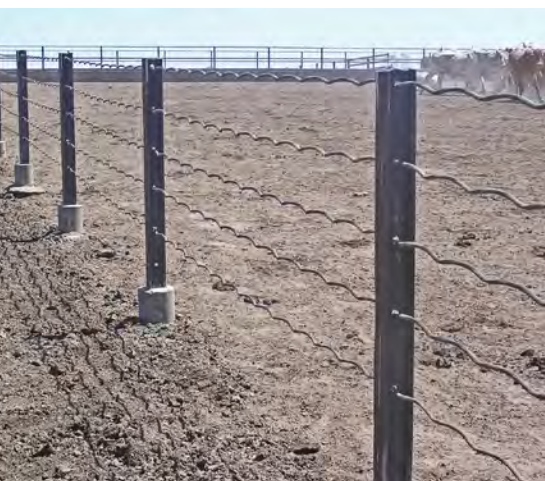
Secondhand or surplus materials from other industries are commonly used e.g. railway line and bore casing.
