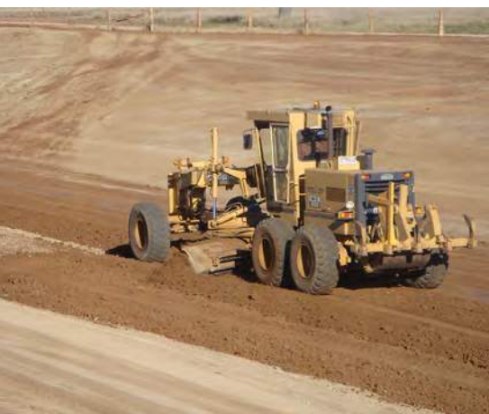
Graders are used for excavation, batters and precision finishing in the final shaping of surfaces (e.g. roads, pens, building foundations).
