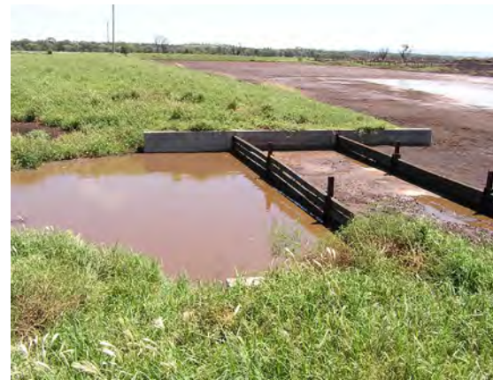
Horizontal timber slat control weir after a storm, with floating material retained in the sedimentation basin.
