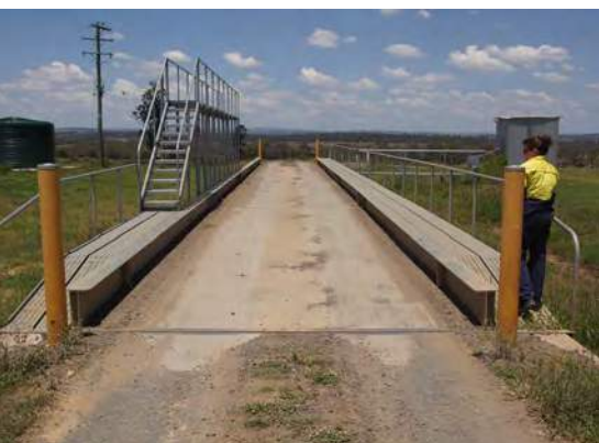
Boldly painted bollards placed at the entry and exit guide the truck driver and protect the weighbridge sides.
