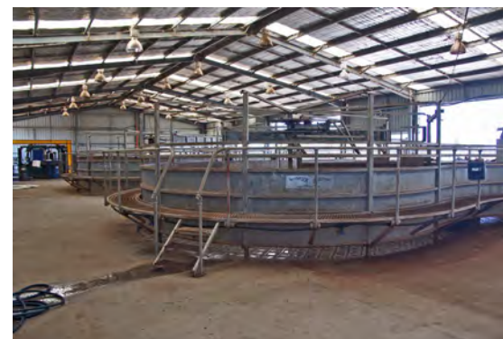
Steel frame building over entire processing area. Lighting is provided with clear roof sheets and artificial lamps.
