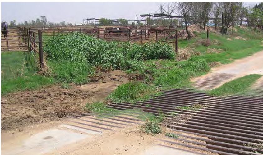
Grid culvert drain crossing makes it difficult to clean under the grid.
