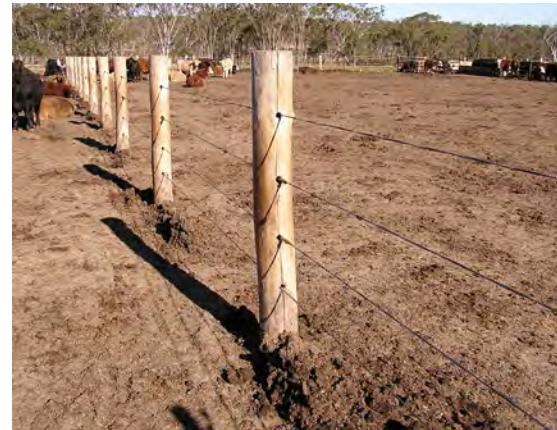
Cables can pass through wooden posts minimising corrosion and cable fraying. This fence line has no top or belly rail.
