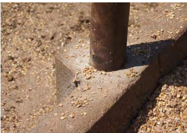
Local thickening of the feed bunk wall is strong but may make cleaning difficult.
