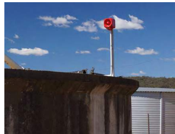
This siren alerts management when water in the tank drops to a critical level.
