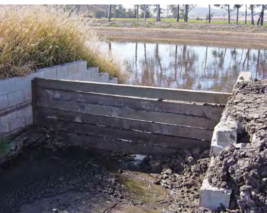
Sediment has built up between the walls of this control outlet as there is insufficient space for maintenance equipment to reach it. The control structure should have been located at the end of the block wall structure.
