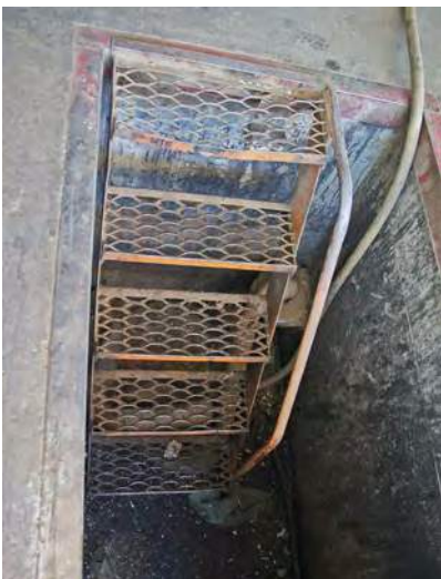
Access to pits should comply with the relevant WHS requirements, with fixed handrails.
