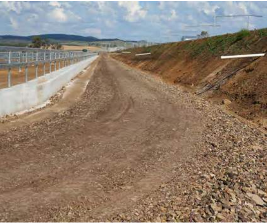
Acceptable limits for cut and fill slopes depend on soil type and strength, geology of the site and saturation.
