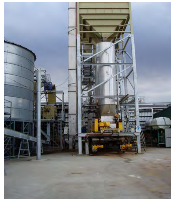
Steam-flaking - grain is transferred to green holding bins above the steam chest. After conditioning in the steam chest, grain enters the flaking mill.
