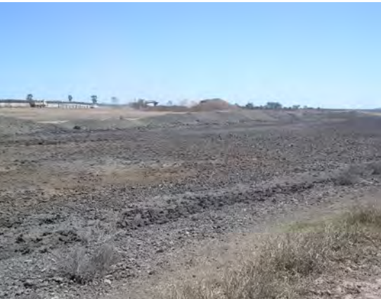
Sediment basin effectively retaining sediment and draining to bed level, allowing deposited solids to dry.
