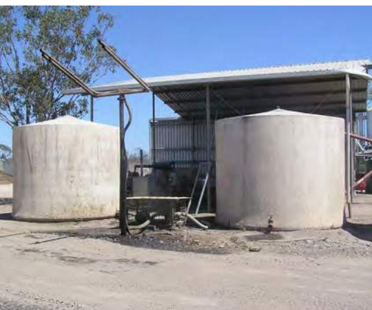
A well-prepared site with a solid foundation for liquid ingredient storage tanks. Flat-bottom concrete tanks are commonly used.
