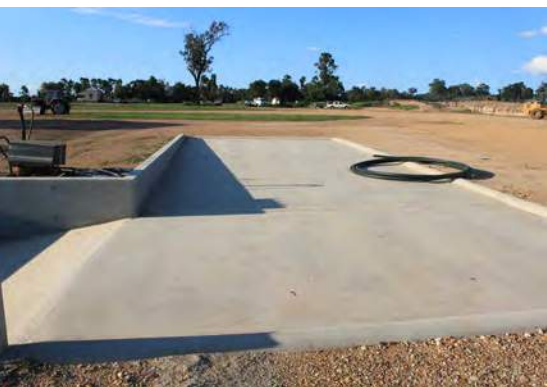
Concrete pad with suitable length and width for most feedlot vehicles, kerbed pad, adequate slope on pad and suitable wastewater collection system.
