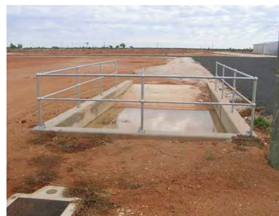
This single trafficable sedimentation basin is adequately sized for cleaning machinery, and has handrails for safety. Wastewater drains to bed level.
