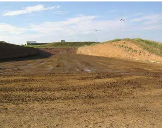
Hillside pits excavated into the side of the slope. The natural slope provides adequate drainage for the open end of the pit.
