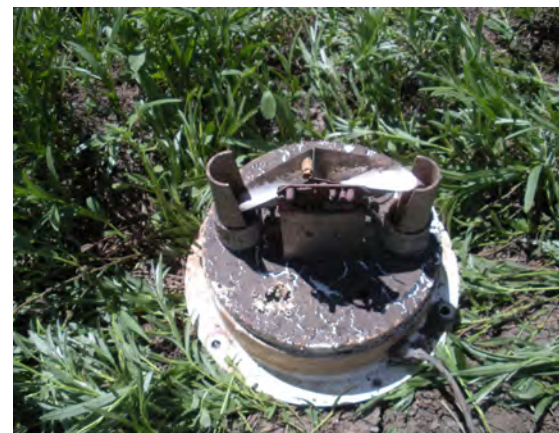
A rain gauge installed in a site subject to stormwater flows. The gauge was inundated and all components had to be replaced.
