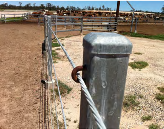
External eyelets hold cables running past steel posts. Hollow posts are capped to exclude water.
