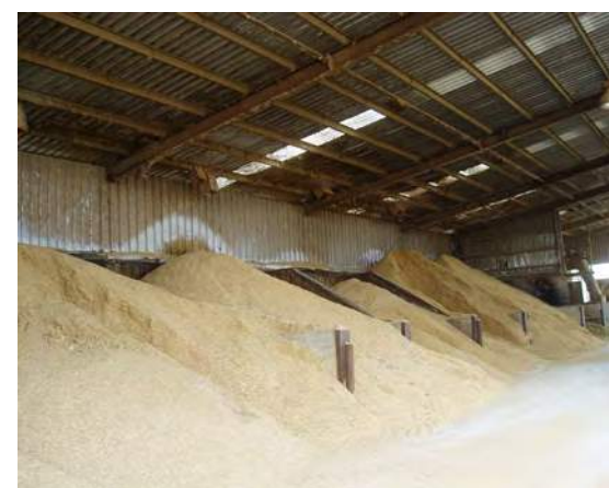
Length and width of individual bays and height of divider walls should be designed to match the volume of material to be stored. Grains with a flatter angle of repose will form flatter piles.
