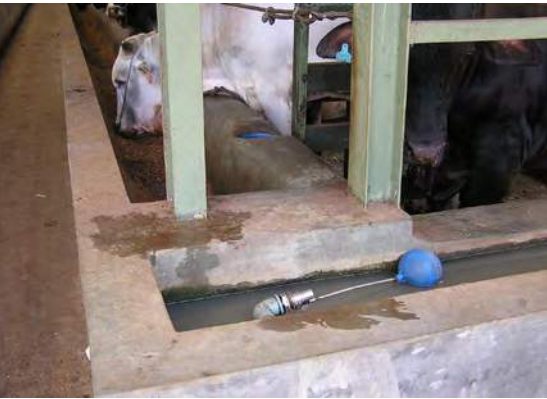
Unprotected floats can be damaged resulting in an overflowing trough and wet spots within the pens.
