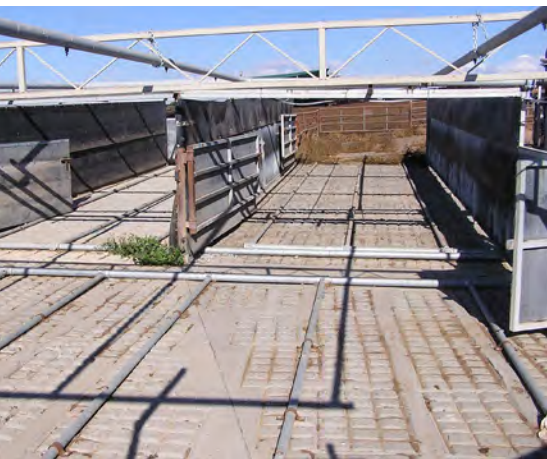
Side by side soaking pens with above-floor pipework and an overhead spray system
