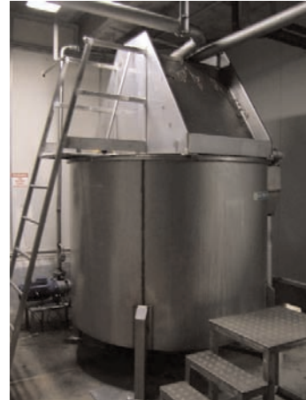
The "white" wastewater catch tank
