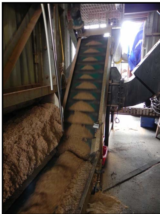
Sawdust feed conveyor system
