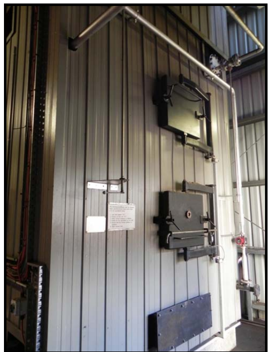
Boiler with inspection doors
