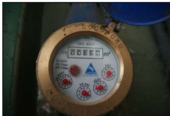
Figure 10 – Water Meter at Wainui Feedlot
