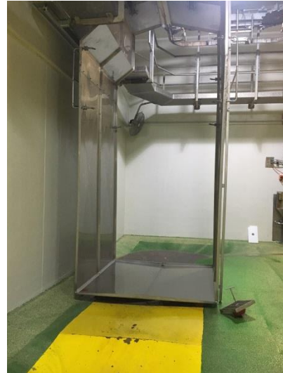
Figure 13: New capture tray and drain
