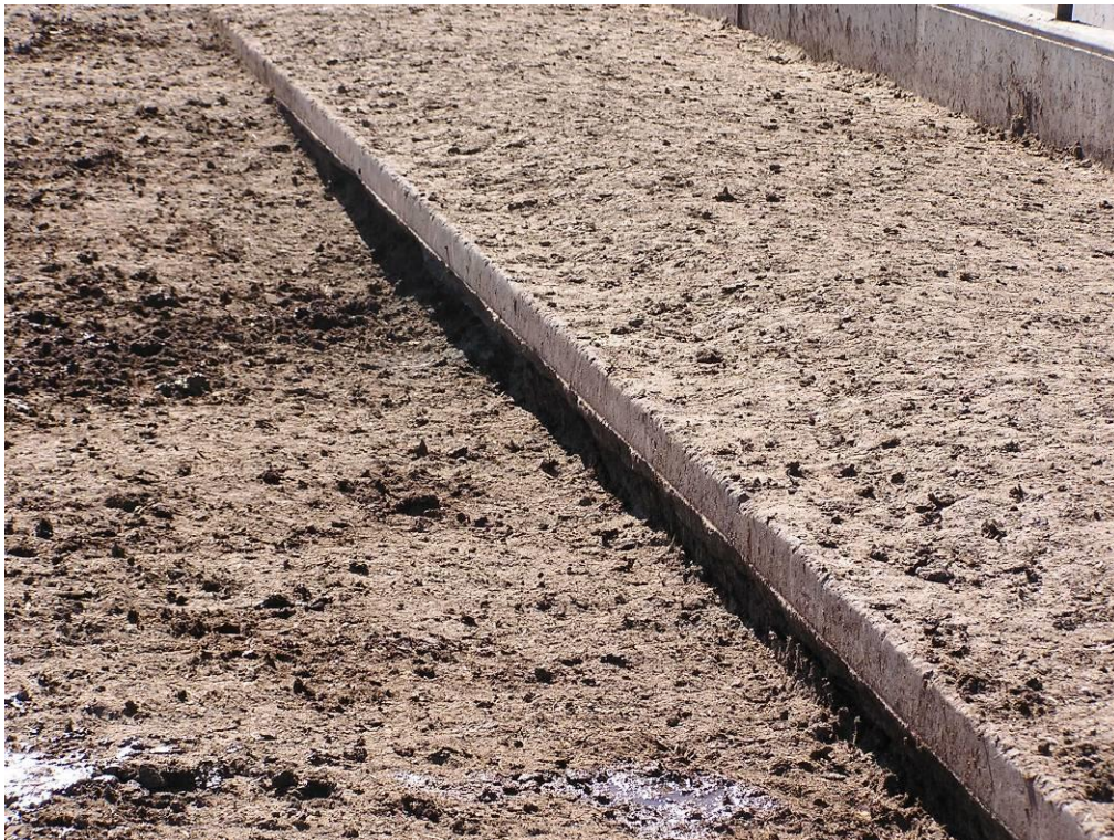
PHOTOGRAPH 48 – PEN SURFACE EROSION BEHIND FEED BUNK APRON
