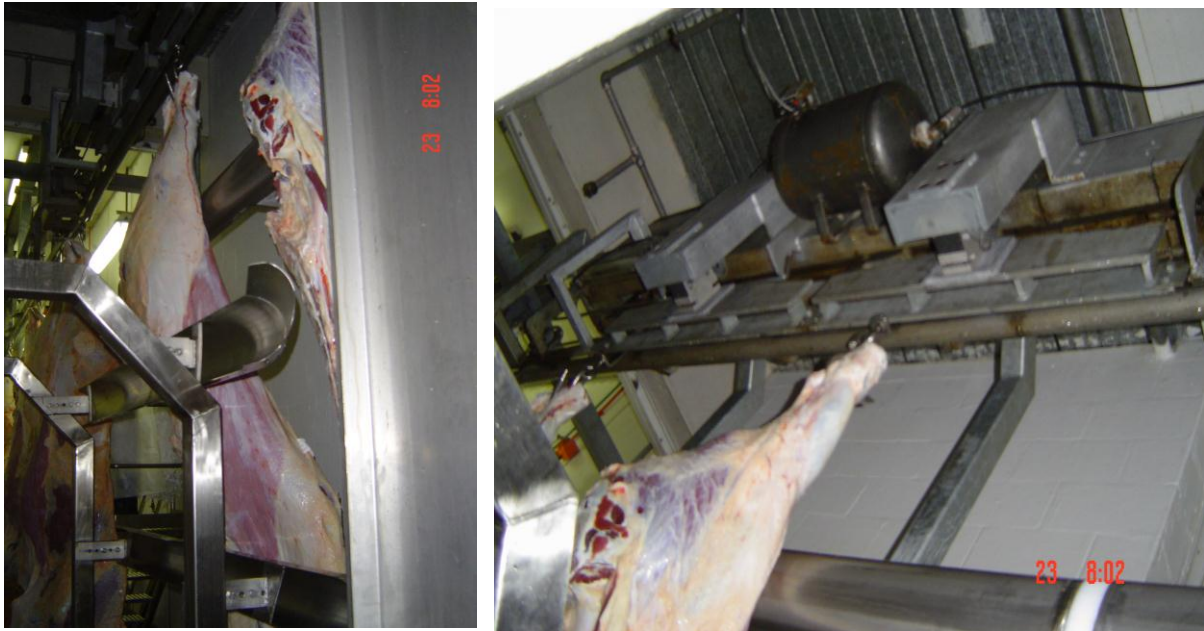
Pictures 1 & 2 – Installation of ALVS at ACC plant showing critical system components including rub bar electrodes, load cells and controller.
