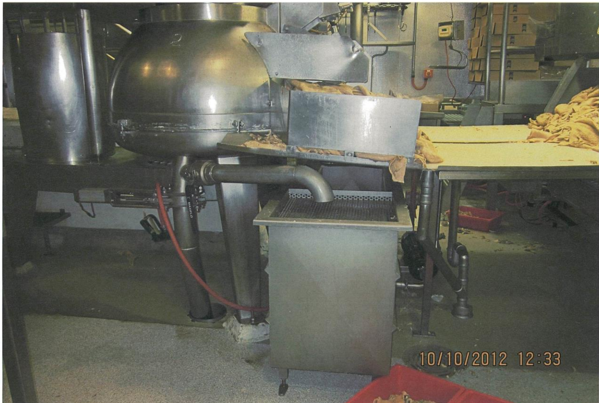
Photo 1: Tripe wash water reuse pilot system in beef processing at a large beef processing plant.
