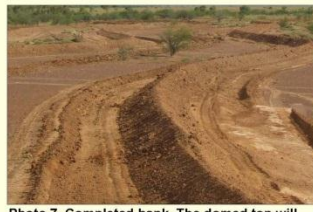
Photo 7. Completed bank. The domed top will allow rainfall to flow away, minimising pooling on bank top.
