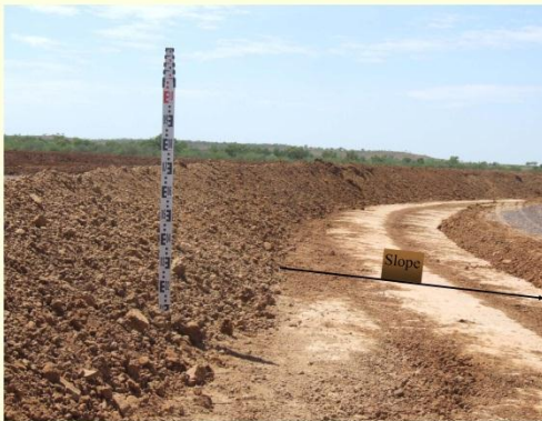
Photo 3. The bank has been constructed to a height of 70 cm. The borrow area slopes away from the bank which is essential. This prevents the grader blade from undercutting the bank.
