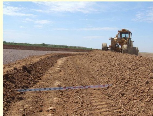
Photo 4. The borrow area is approximately 2 m wide. During construction one wheel of the grader will run along the base of the bank, the other wheel will run on undisturbed soil above the borrow area (see wheel tracks).
