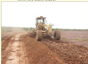
Photo 6. Taking second blade of soil (rolling onto existing bank) on inside of pond.
