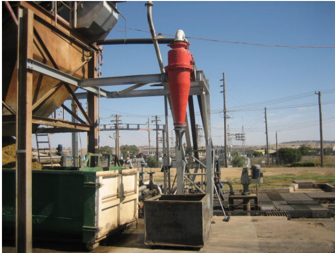
Figure 3. Hydrocyclone mounted on support structure showing bin for grit collection
