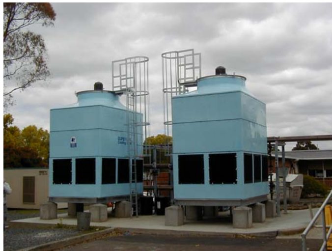
Figure 5. Induced draft cooling tower.
