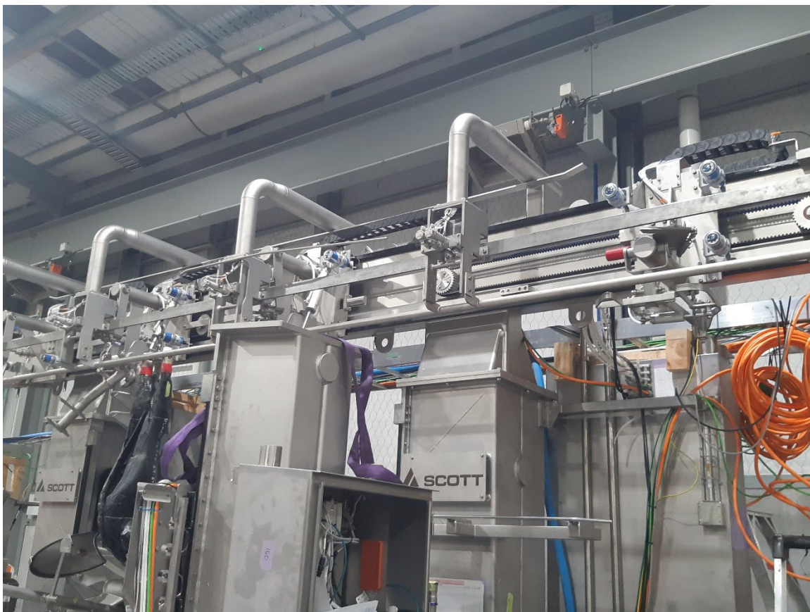
Figure 25: LEAP III Transfer station showing electro-mechanical lubrication mounting arrangement.
