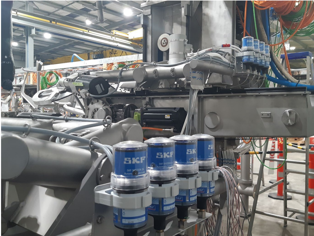
Figure 22: LEAP III Forequarter station Examples of adaption concepts throughout the cutting heads.
