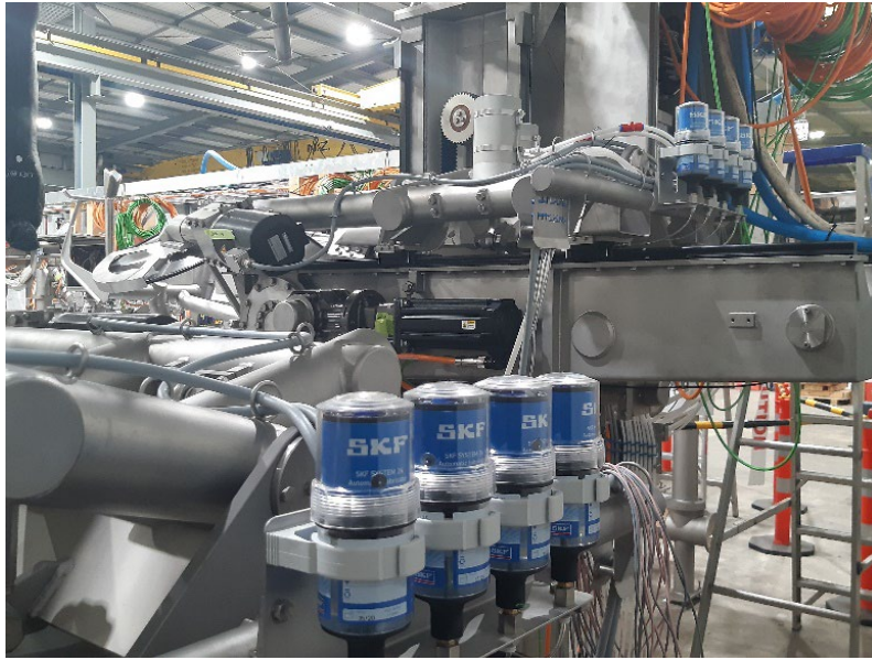
Figure 23: LEAP III Saddle station Examples of adaption concepts throughout the saddle cutting heads.
