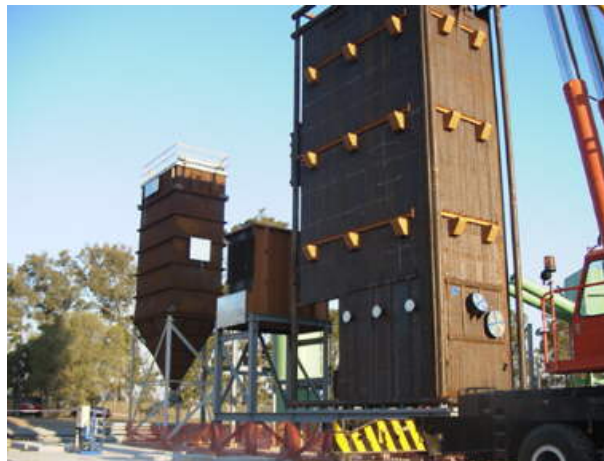
Figure 4 Fluidised bed combustion unit installed on green waste to energy site in Staplyton, Queensland
