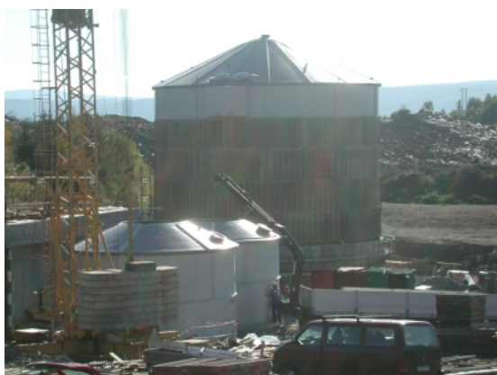
Figure 11 Storage for liquid carbon source and digester
