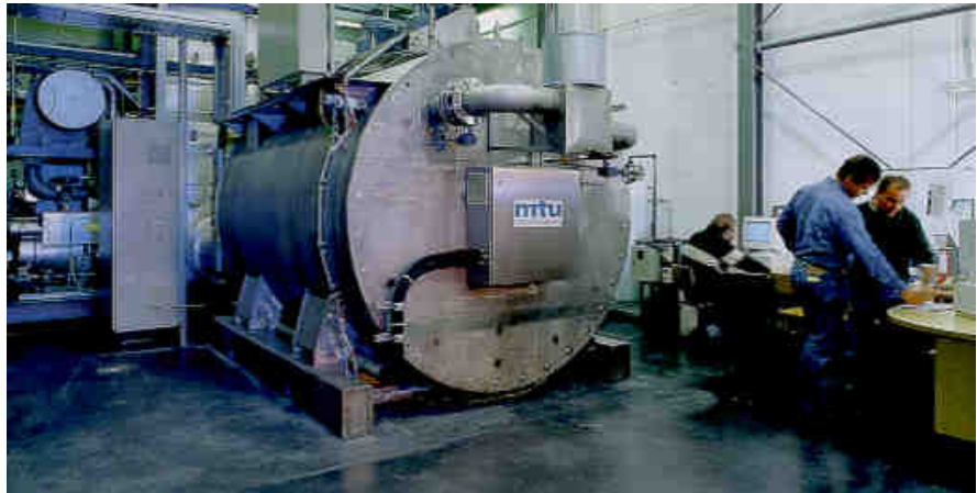
Figure C2 Molten carbonate fuel cell power plant
