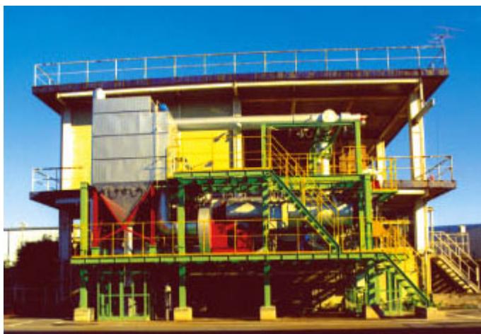
Figure 15 Pyrolysis system for municipal and industrial wastes at Honmoku Factory in Yokohama, Japan
