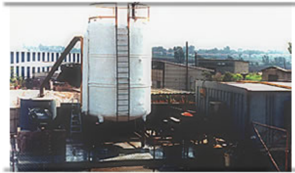
Figure 8 Anaerobic Methanogenic Thermophilic Digestion Unit
