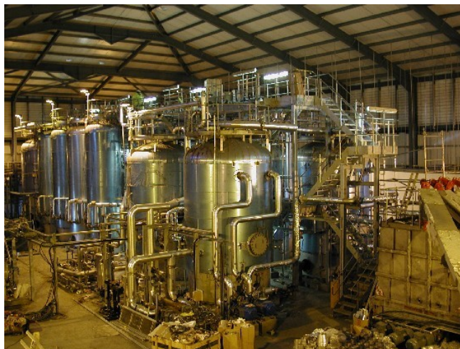
Figure 13 Cambi Thermal Hydrolysis Plant, Dublin
