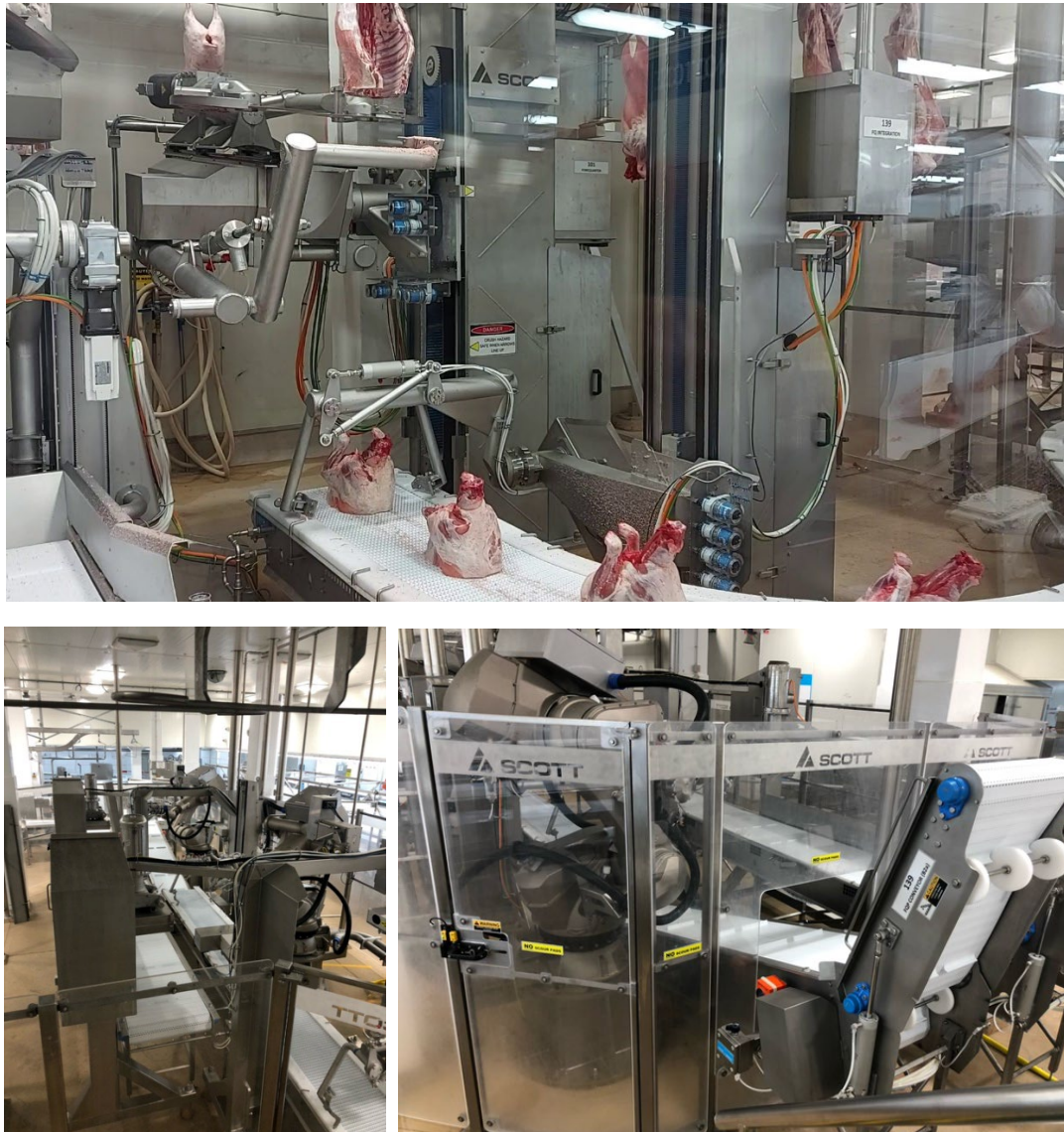
Figure 22: System installation being used for demonstration of the upgrade kit components in production environment.
