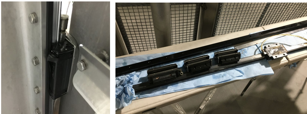
Figure 7: Example of Vertical carriage tracks are found to have suffered distortion and excessive wear.
