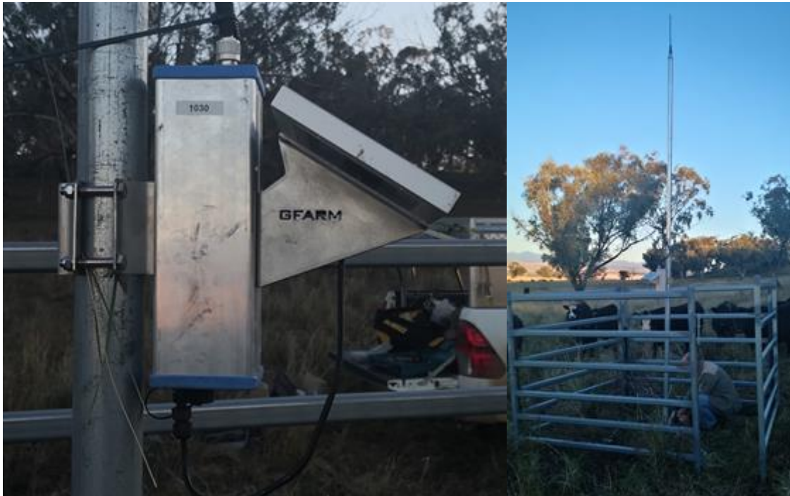
Figure 2: Base Station Installation
