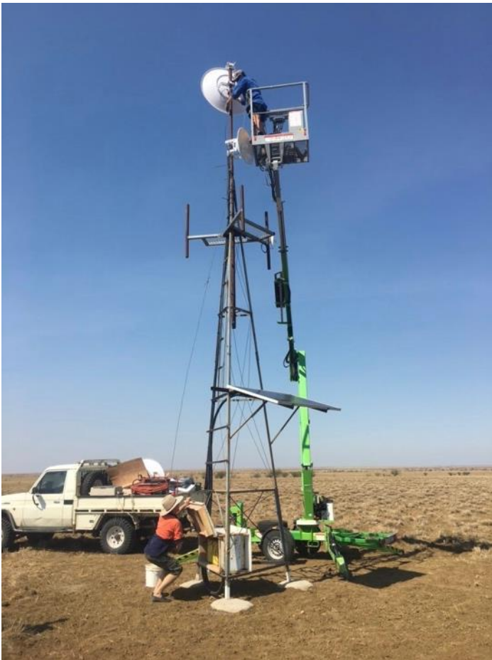
Photo 4: Final alignment of dish commissioned on the Tweedsmuir tower pointing towards Essex.
