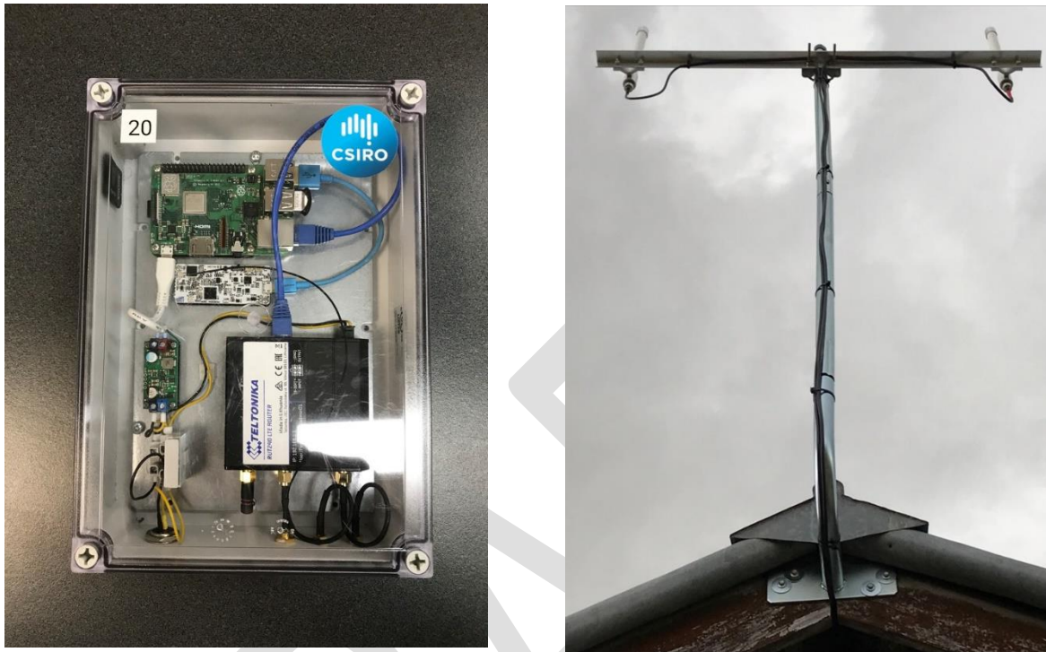
Figure 14. Pictures of the gateway and LoRa antenna installed at the trial sites
