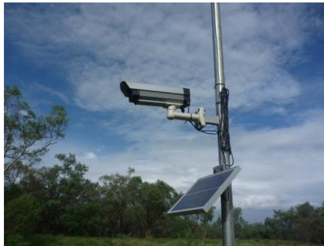
Figure 8 Harrington System's remote camera for the Next G network
