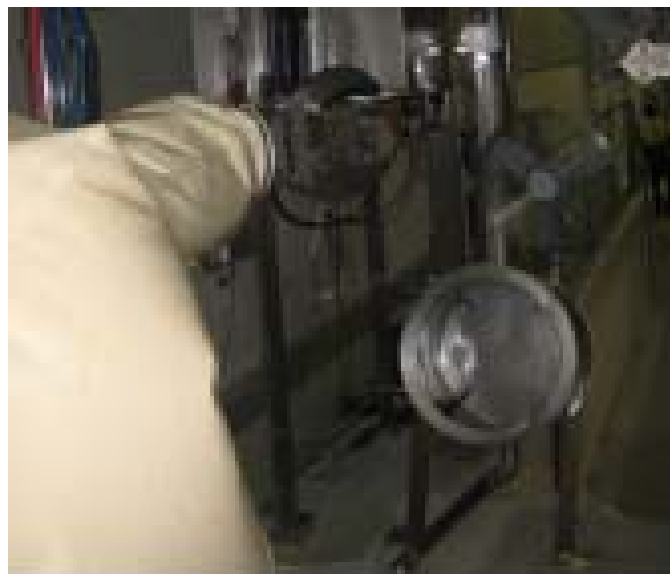
Figure 22 – Original Wash tank Position
