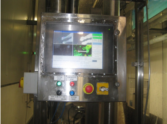
Figure 2 - HMI Cabinet with Robot Isolator, E-Stop and Fortress Lock
