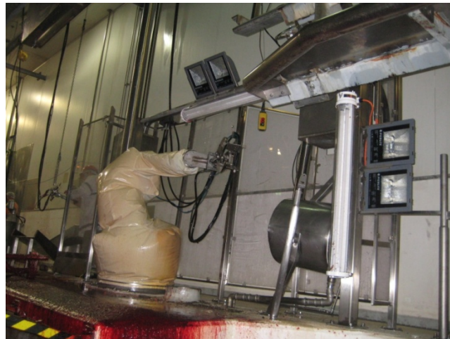
Figure 25 – Cell Enclosed by guarding
