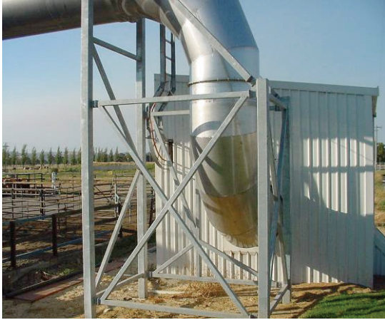
The Biofilter Fan Shed
