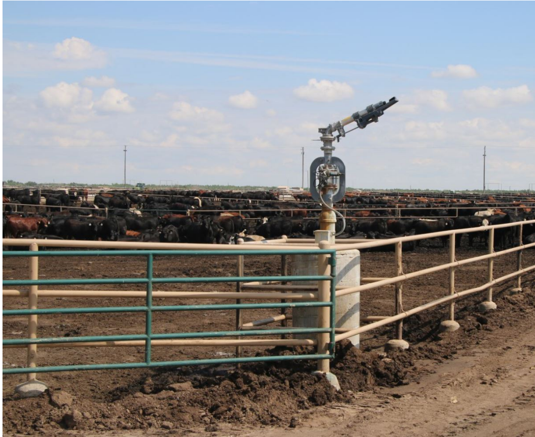
Photograph 12 – Solid-set sprinkler in feedlot pen
