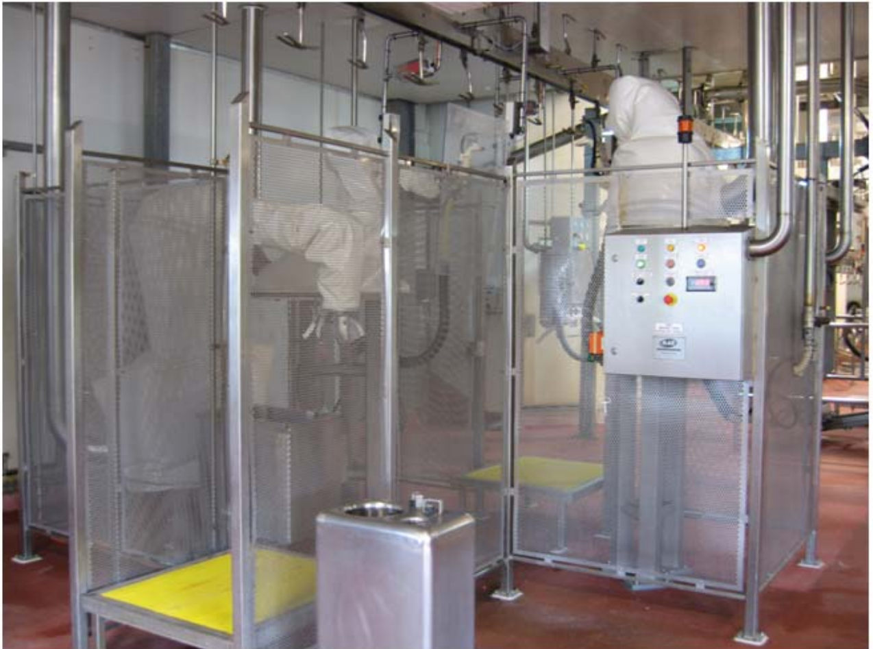
Fig. 3 Cell Perforated guarding installed at GMP
