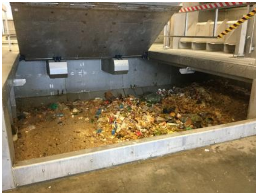
Raw Waste Bin
