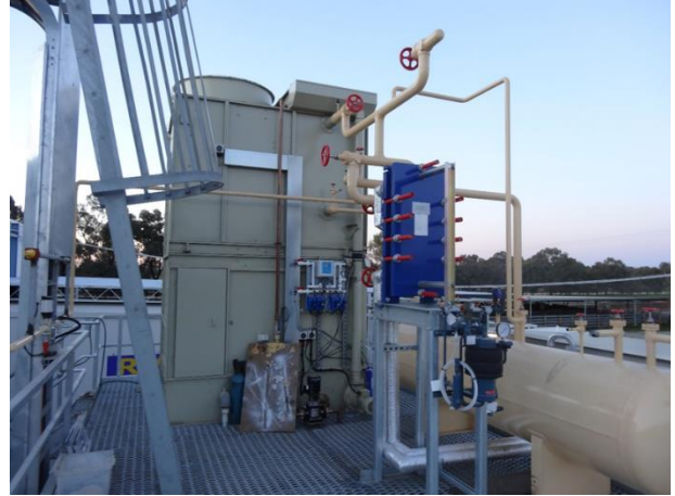
Figure 12 - Evaporative Condenser, plate heat exchanger for Heat recovery and Liquid Receiver
