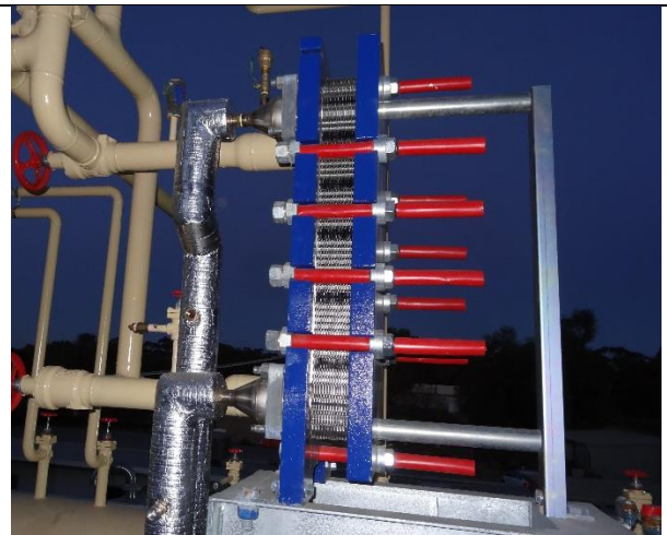
Figure 18 - Heat Recovery Plate Heat Exchanger
