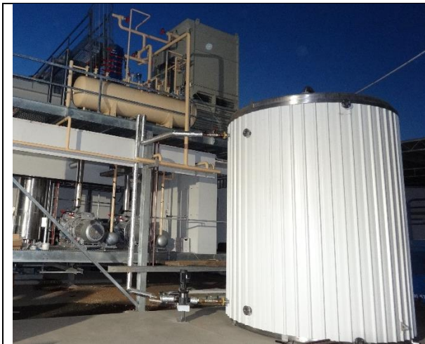
Figure 17 - Hot Water Tank
