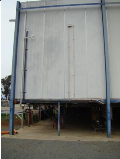
Figure 6- Uninsulated Suction Gas and Liquid Lines to Load Out Chiller
