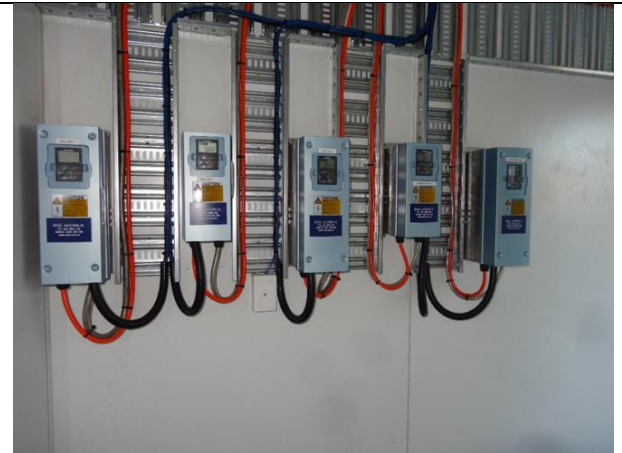
Figure 14 - VSD for evaporator fans
