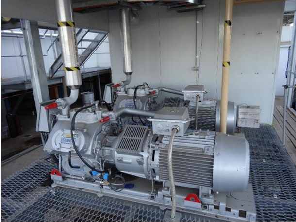
Figure 11 - High and Low Stage Reciprocating Compressors
