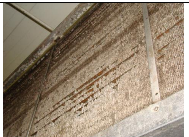
Figure 5 - Degraded Evaporator in Big Lamb Chiller
