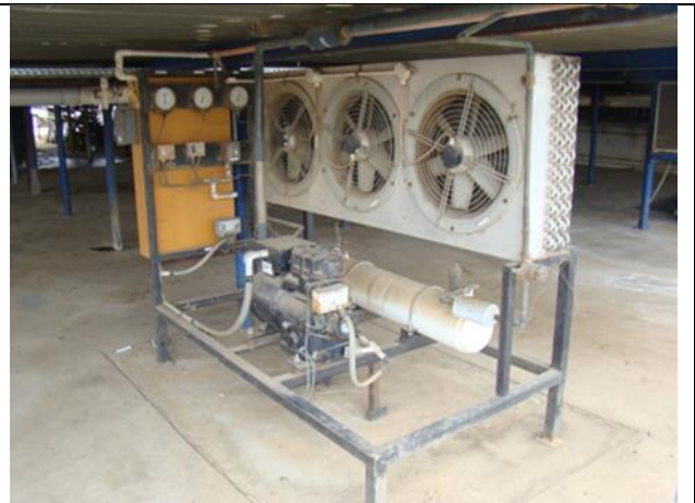
Figure 3 - Condensing unit for Load out Chiller, installed underneath the chiller
