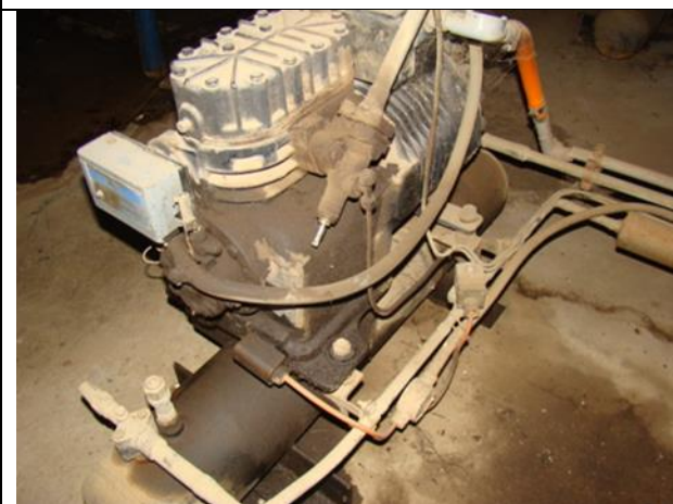
Figure 4 - Oil leaks at the compressor - often a sign for refrigerant leakage
