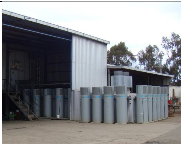
Figure 8 - R134a Heat Pumps
