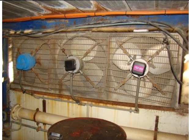
Figure 7 - Old condenser Coils with Minimal Fan Staging Control
