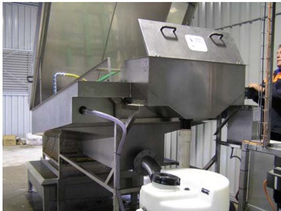
Figure 3: Baleen filter installation
