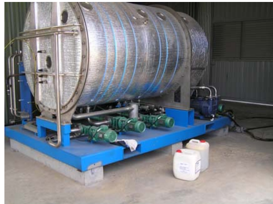
Figure 4: Distech D-1003 installation
