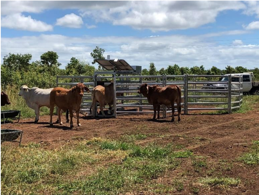
Figure 3. Walk over weigh installation at water point to improved pasture paddock.
