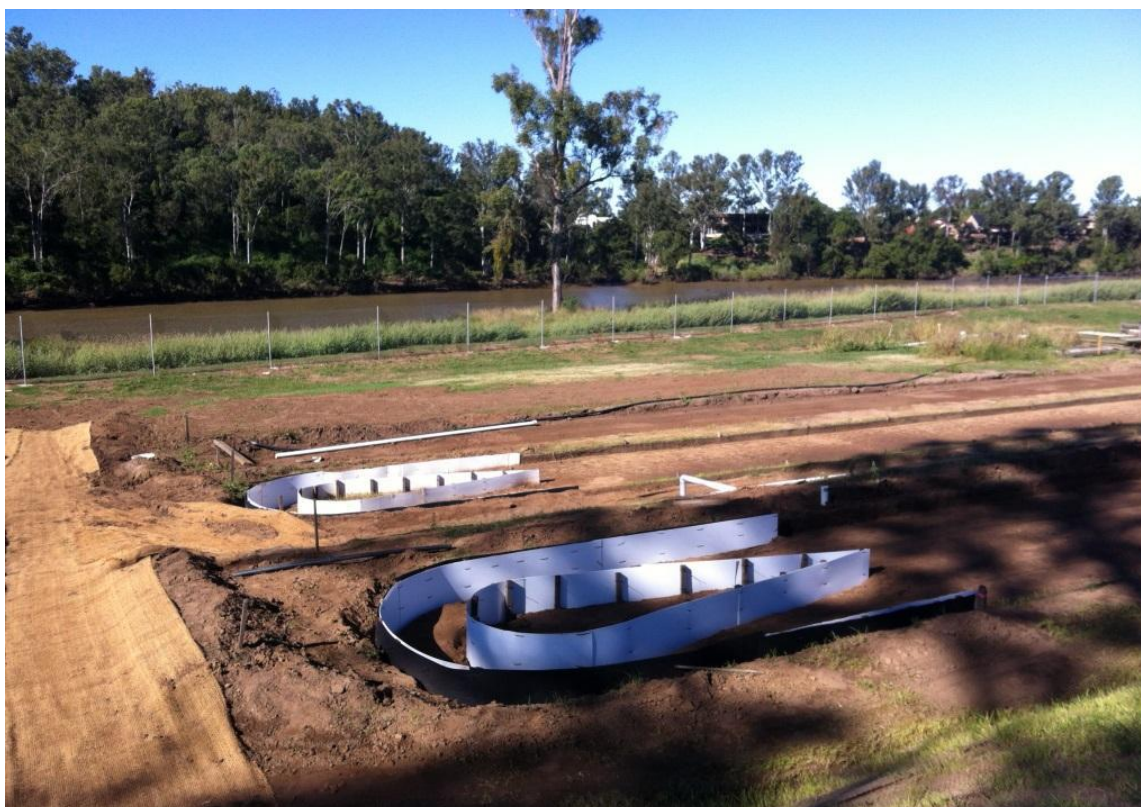
Fig. 2. Construction of 40,000 L raceway ponds during the first phase of the microalgae farm project in March 2013.
