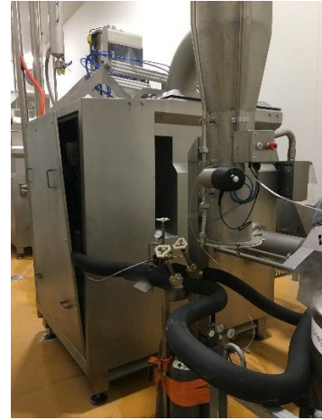
Nitrogen supply lines to mixer manifold
