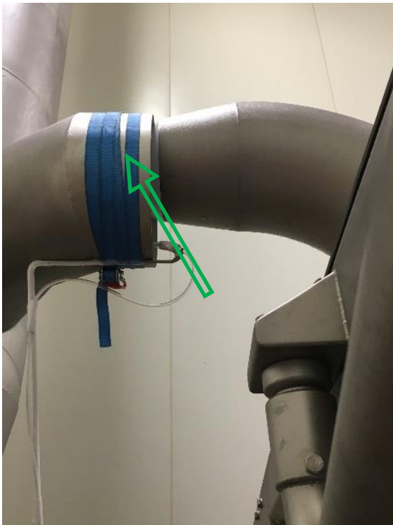
Photo 9: Nitrogen gas vented from mixer to exhaust system.
