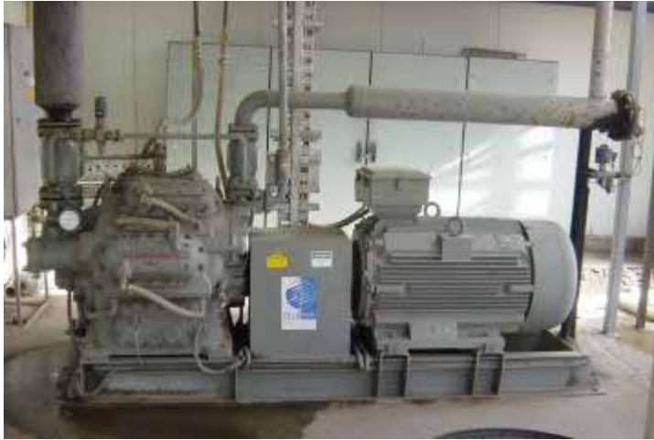
Refrigeration compressors are high energy consumers
