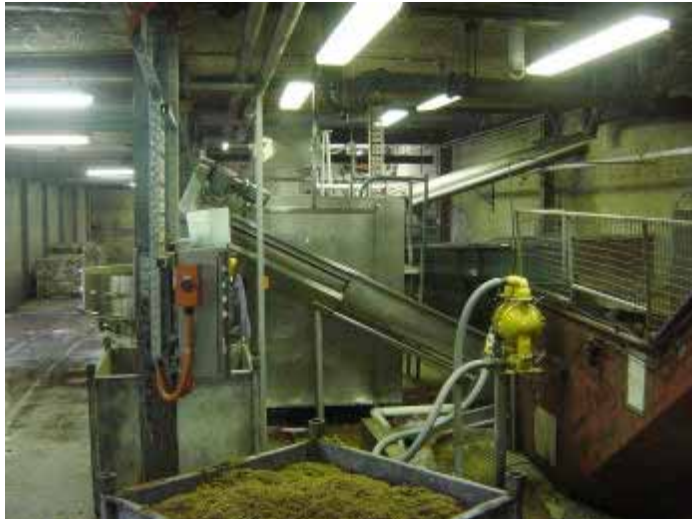
Dewatering screw system
