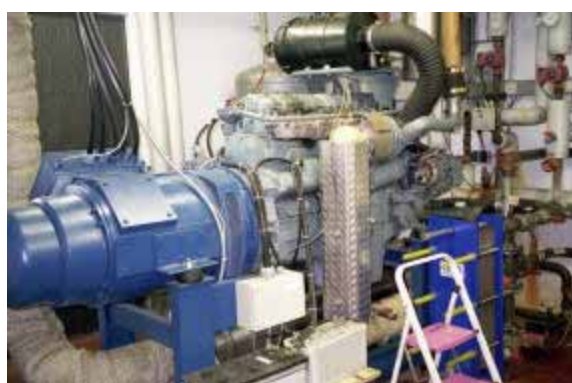
Gas engine, running on biogas
