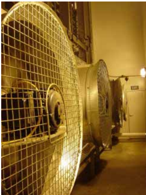
Blast chiller fans
