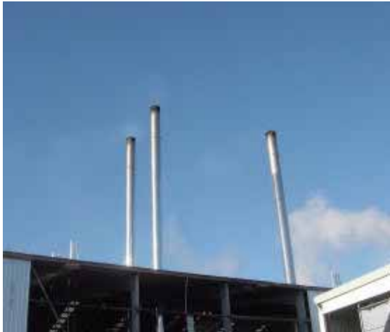
These boiler stacks are one example of a point source
