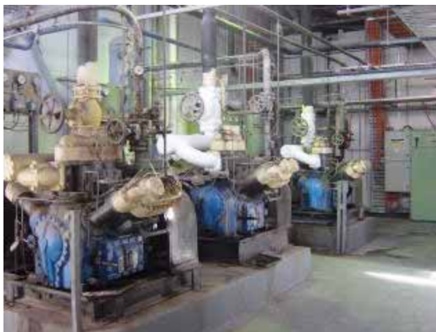
Refrigeration plant room
