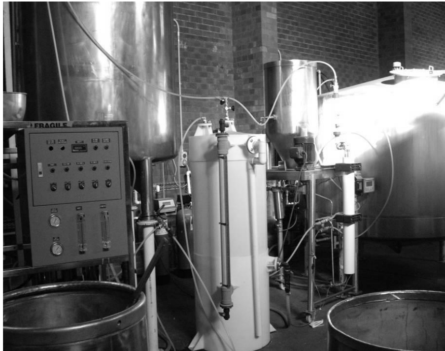
Figure 4: Water Purification System, including two reverse osmosis units.
