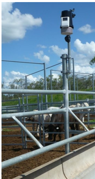
Figure 1 Automated weather station.
