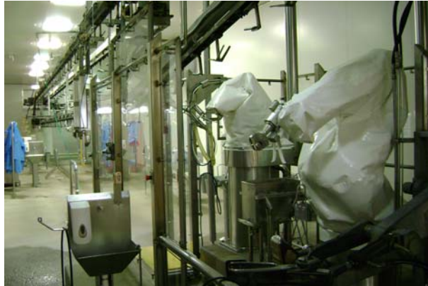
Figure 4 Robot cell with protective guarding
