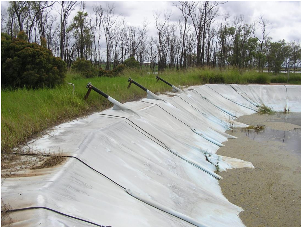
PHOTOGRAPH 16 – SLUDGE EXTRACTION PIPELINES (DEFLATED POND COVER)
