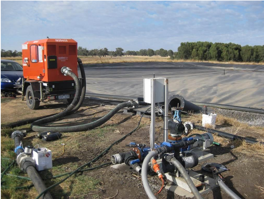
PHOTOGRAPH 42 – VACUUM PUMP AND PIPEWORK
