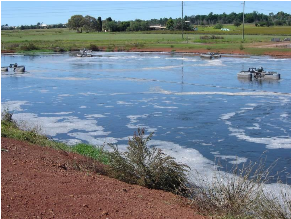
PHOTOGRAPH 4 – MECHANICALLY-AERATED AEROBIC POND
