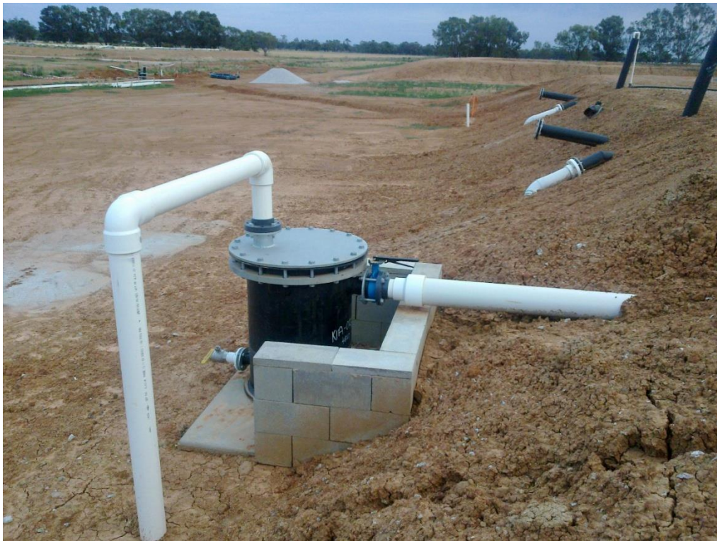
PHOTOGRAPH 18 – SLUDGE (BLACK) AND EFFLUENT (WHITE) REMOVAL PIPES
