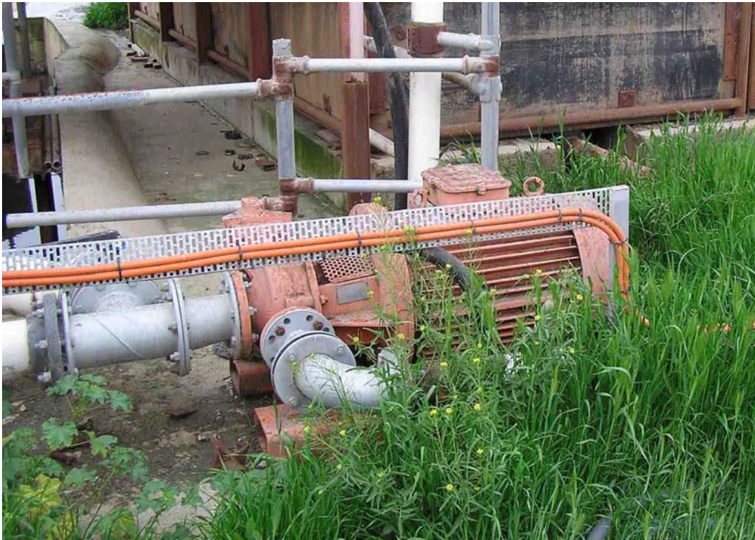
Photograph 9 – Water supply pump
