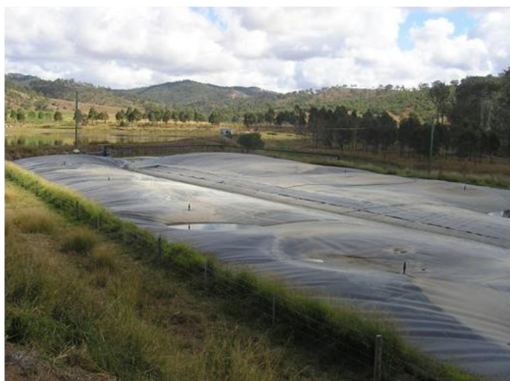
Figure 10 – Covered anaerobic pond (CAP)
