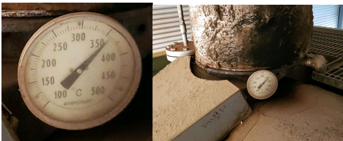
Figure 34: Boiler stack temperature
