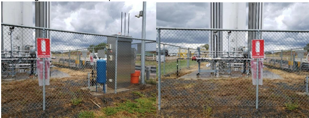
Figure 8: LNG compound and metering point
