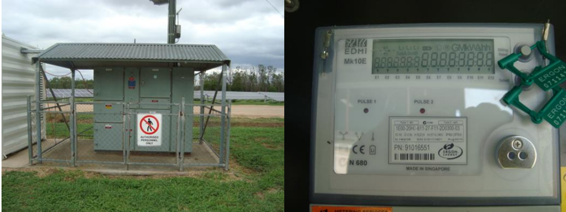
Figure 7: Mill plant electricity meter
