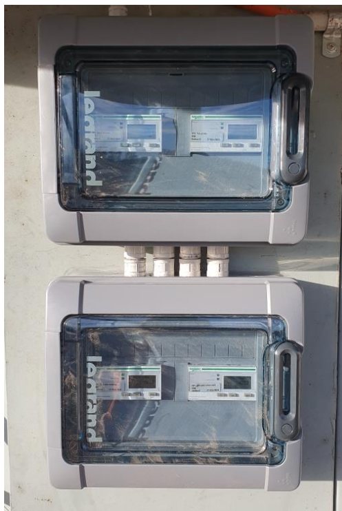
Figure 20: Main switchboard electrical meters
