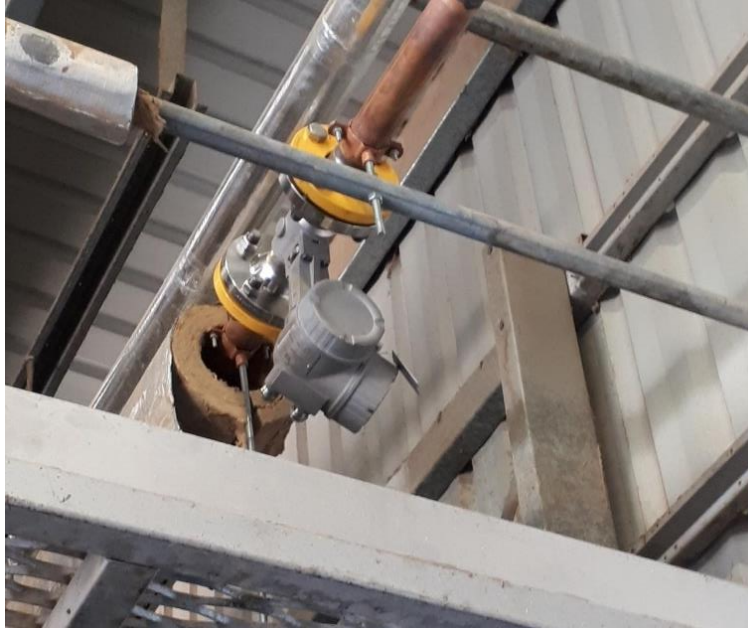
Figure 18: hot well steam supply meter
