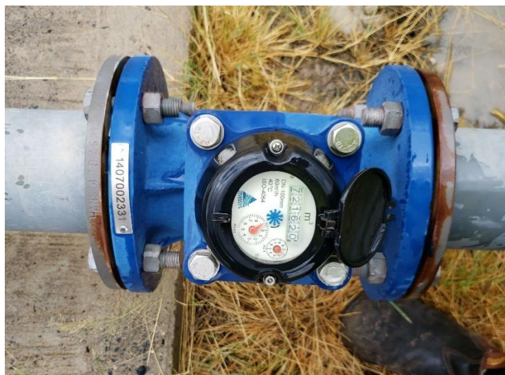
Figure 6: Bore 2 - water meter
