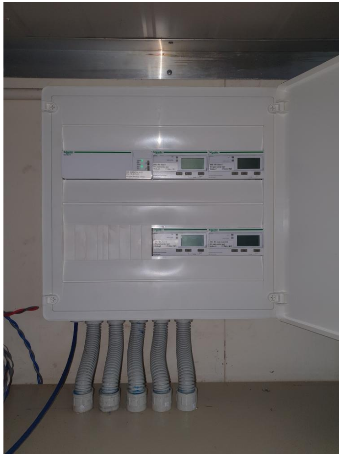
Figure 19: Mill motor electricity meters
