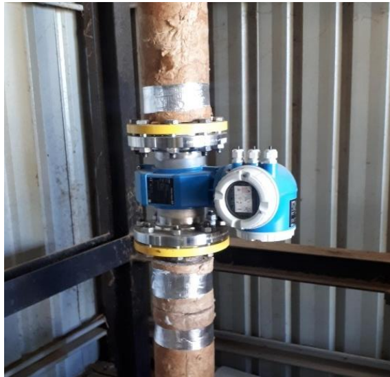
Figure 14: boiler feedwater meter
