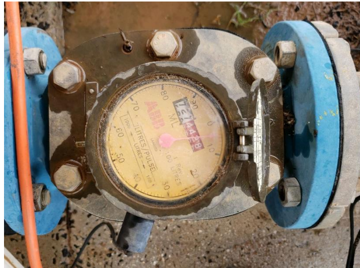
Figure 5: Bore 1 water meter
