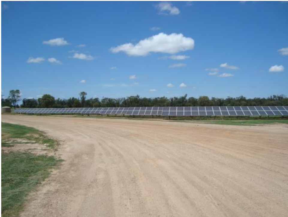
Figure 2: Existing 300kW p Feedlot ground mount solar PV array
