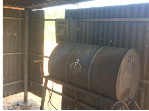
Figure 52 – Fuel storage tank at a remote pumping station.
