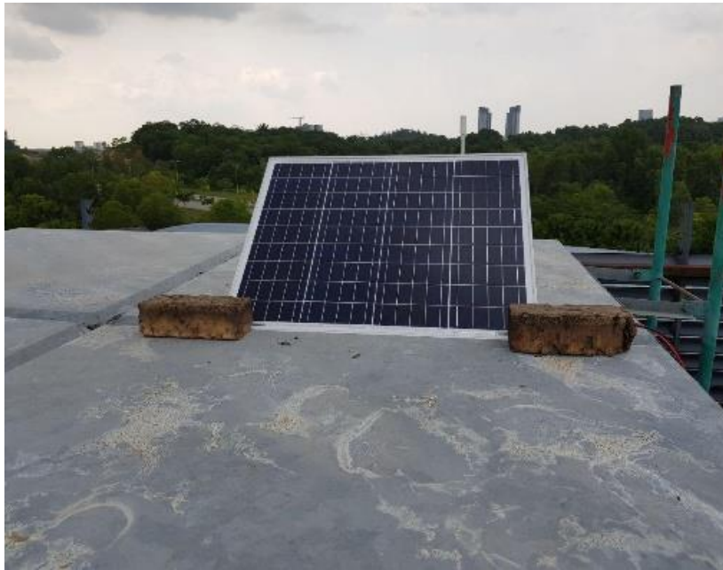
Fig. 53: Solar panel on water tank facing on sunrise direction with 45-degree angle
