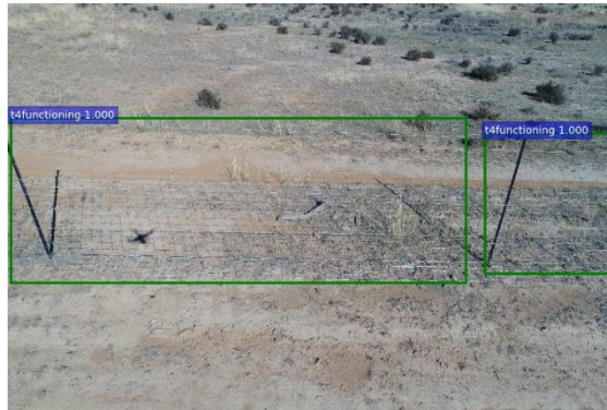
Fig. 47: Type-4 functioning with no damaged fence
