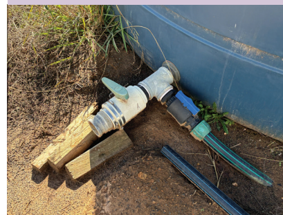
Flat bottom tank
