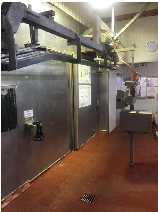
Raised rail height on Production Floor. Push Ram was modified and steel guide Fabricated.
